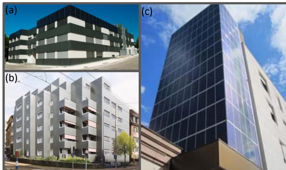
Figure 9. (a) Southwest view of the building after the retrofit, reproduced with copyright permission from [140]. (b) Renovation of a residential building in Zurich, reproduced with copyright permission from [145]. (c) Picture of the BIPV system installed in Bolzano, reproduced with copyright permission from [138].
