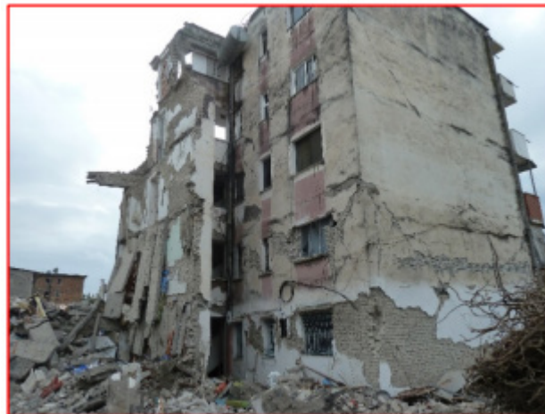
Figure 2-9 Structural damage (source (Lekkas, Mavroulis, Papa, & Carydis, 2019))
