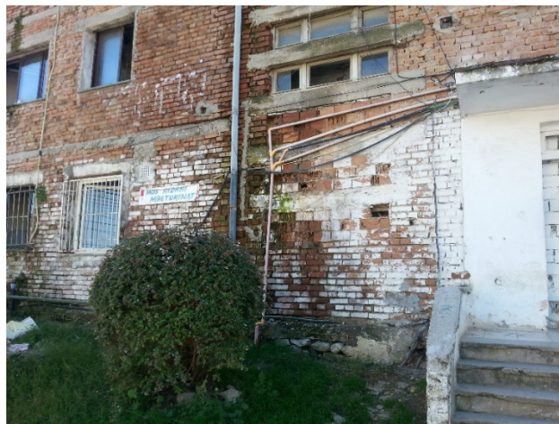
Figure 1-1 Wall deterioration as a result of material degradation (Source: photo by author, Tiranë)
