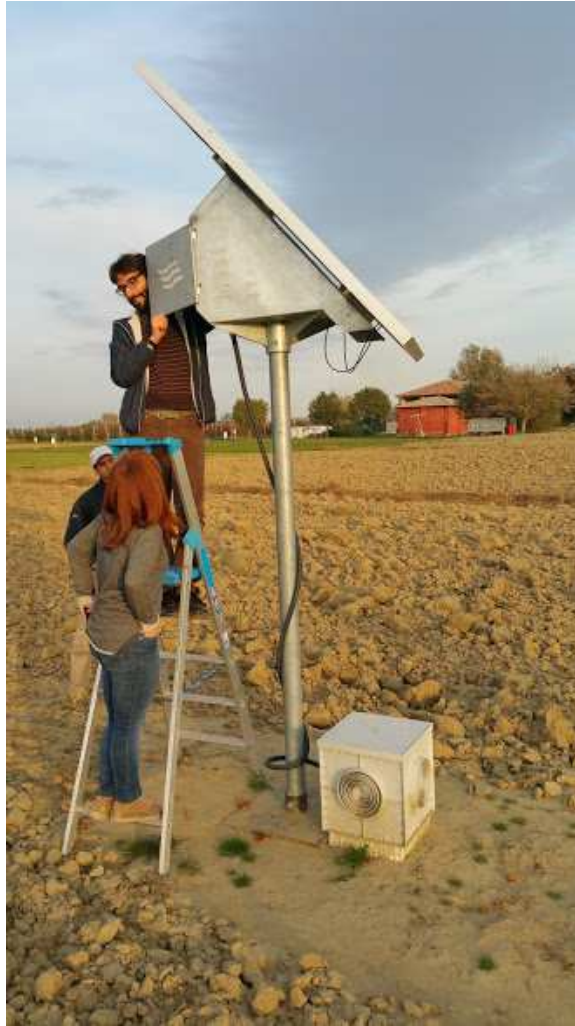
Figure 6.9: installation of NaI(Tl) spectrometer inside the gamma station
