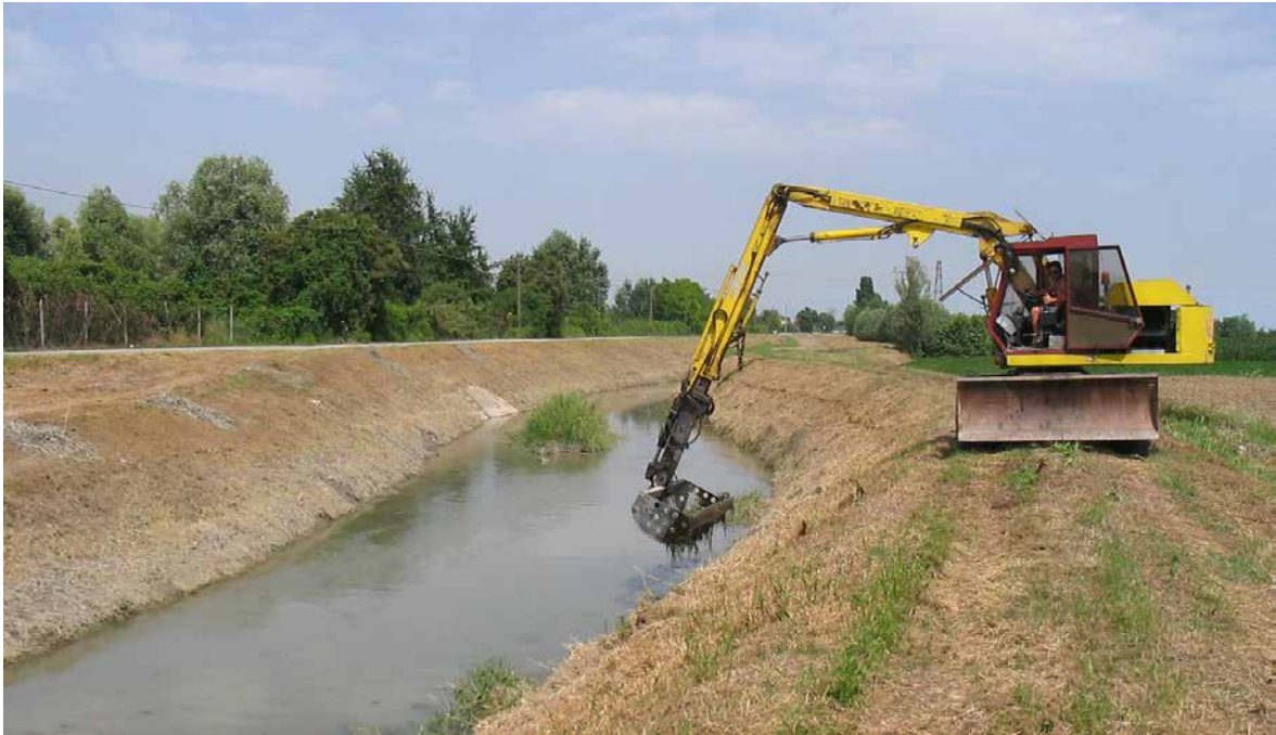
Figure 2.62: The maintenance works along a drainage canal regulate the dimensions and the shape of banks in order to allow machines' movements. (Source: CBRO Consortium)
