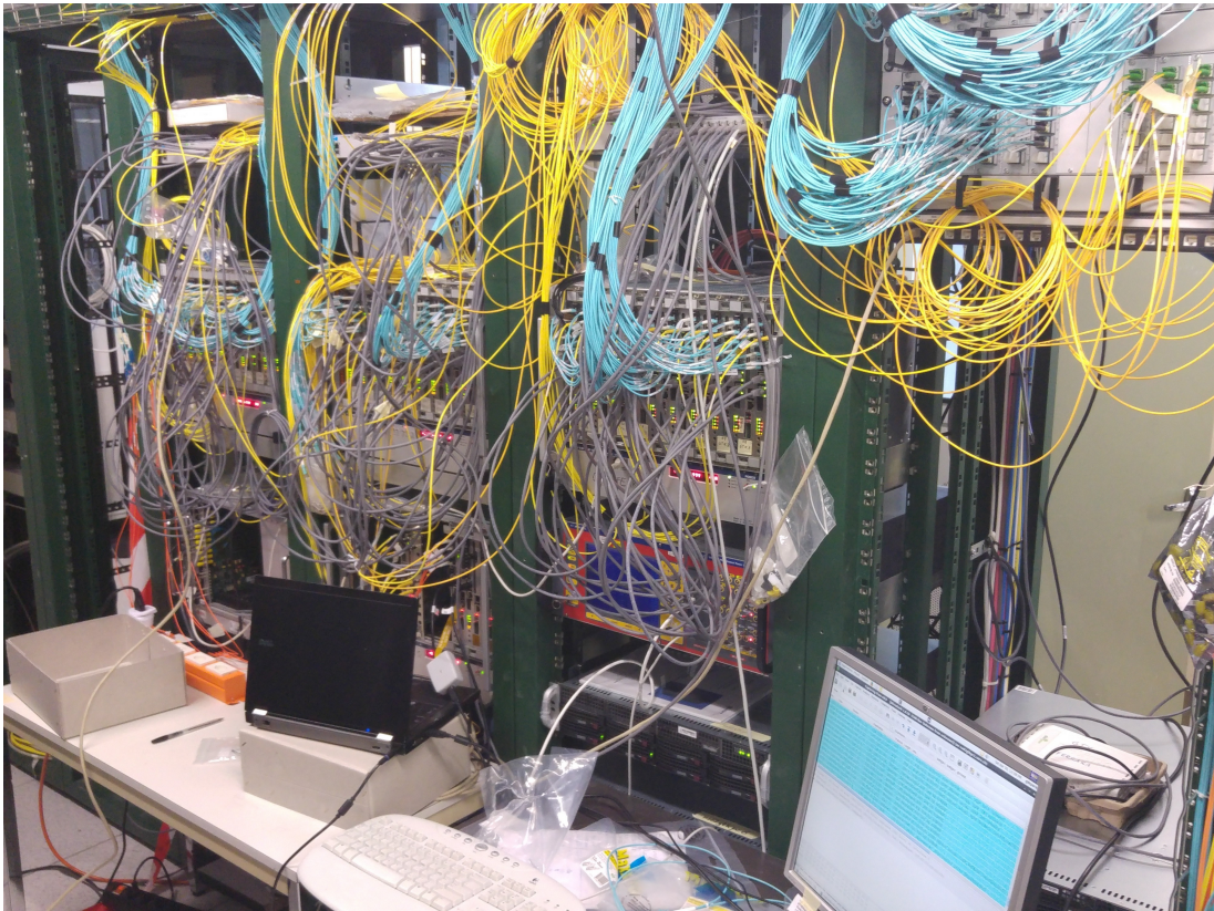
Figure 4.9: The complete GigaTracker data acquisition hardware installed in the PC Farm room at NA62 (August 2016).
