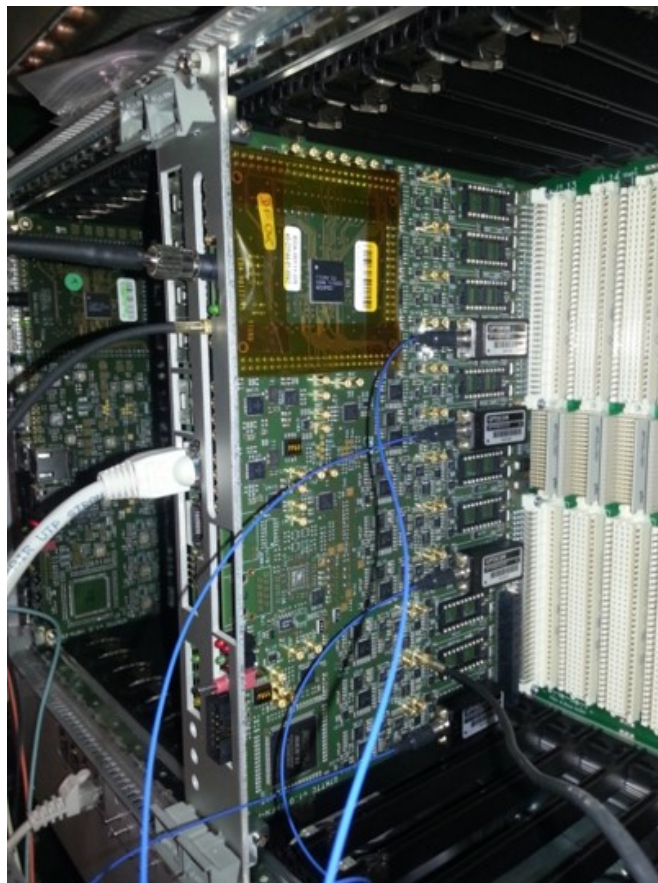
Figure 3.14: A GTK-TTC board installed in the VME crate.
