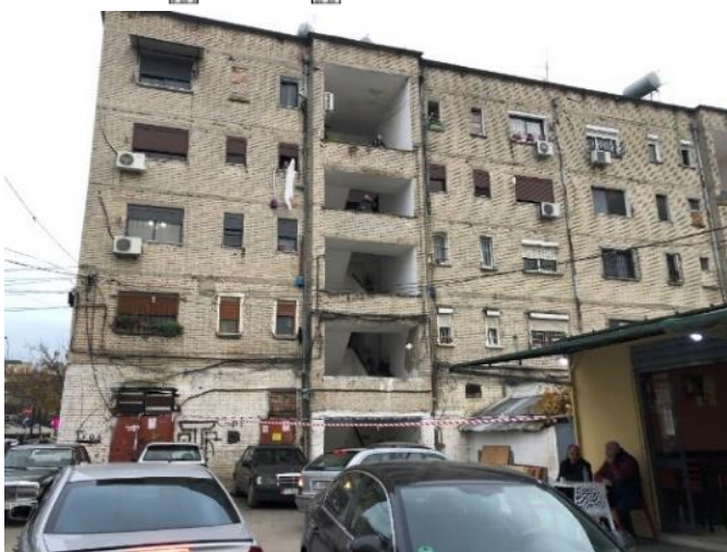
Figure 6 Plan and elevation view of the building type 77/11 and Photo of the building
