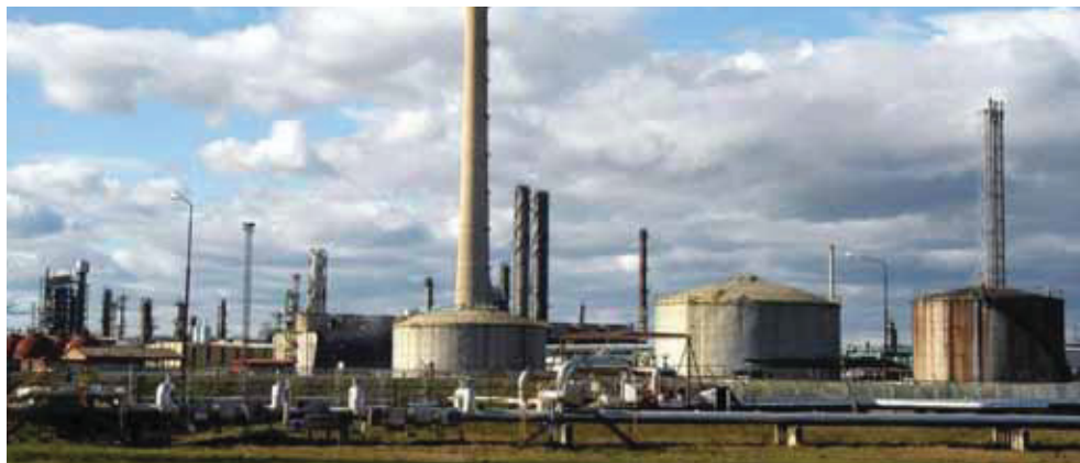
Fig. 66 MOL Sisak oil refinery (source: www.tportal.hr )
