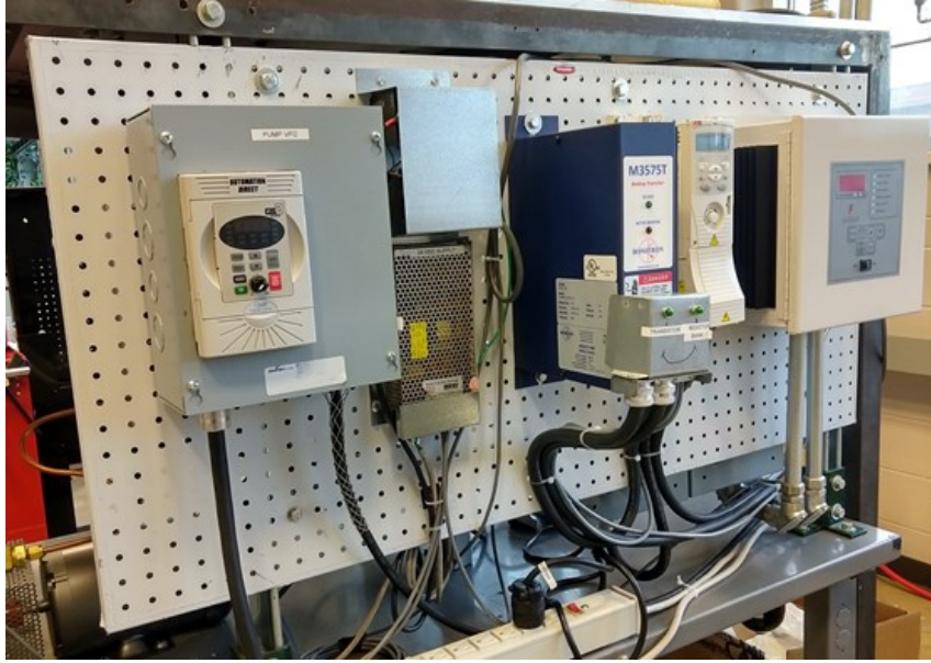
Figure 27: from the left: pump motor inverter, 24 V DC power supply, braking transistor, expander motor inverter, heat torch controller
