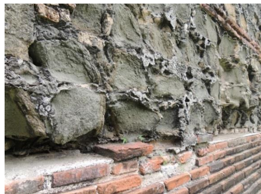
Figure 1.2.1.5 Walls of one of the structures belonging to the complex "Casas Reales" showing the erosion due to the sea waves action.
