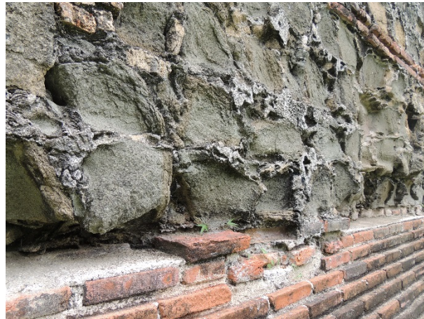
Figure 2.1.1. 37. Effects due to the marine erosion.
