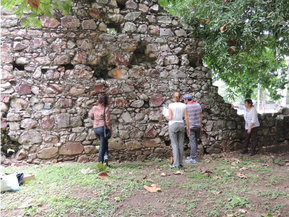
Figure 2.1.1. 30. Wall near the Casa Terrín, showing a reddish chromatic alteration.
