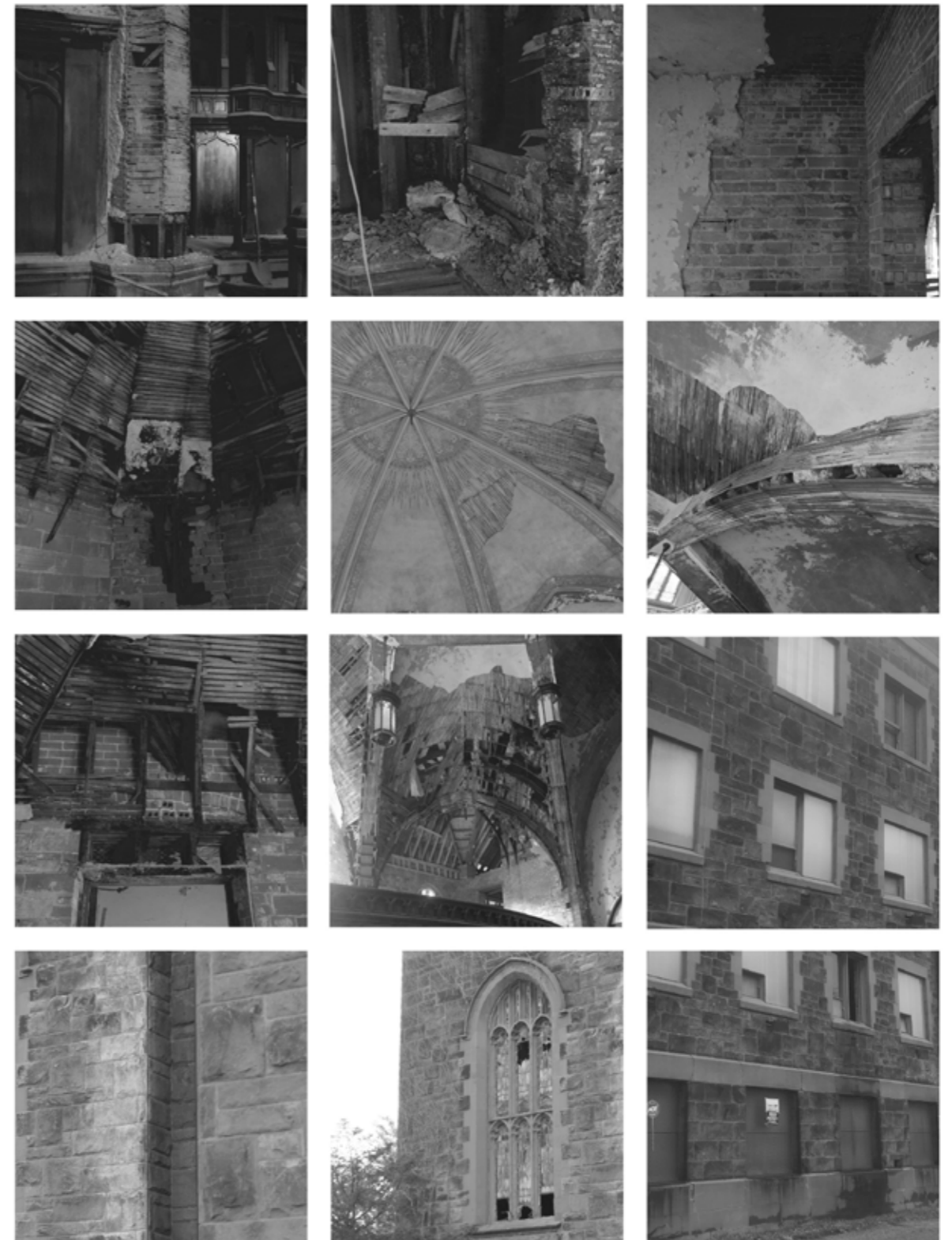
Fig. 7.14 Some of the degradation identified in the Woodward Avenue Presbyterian Church, through the photographic survey of the exterior and interior environments. Among others, shortcomings emerge in vaulted structures and in glass surfaces, masonry gaps, surface deposits in internal surfaces and detachment of internal finishing plaster.
