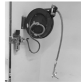
compressed air system
