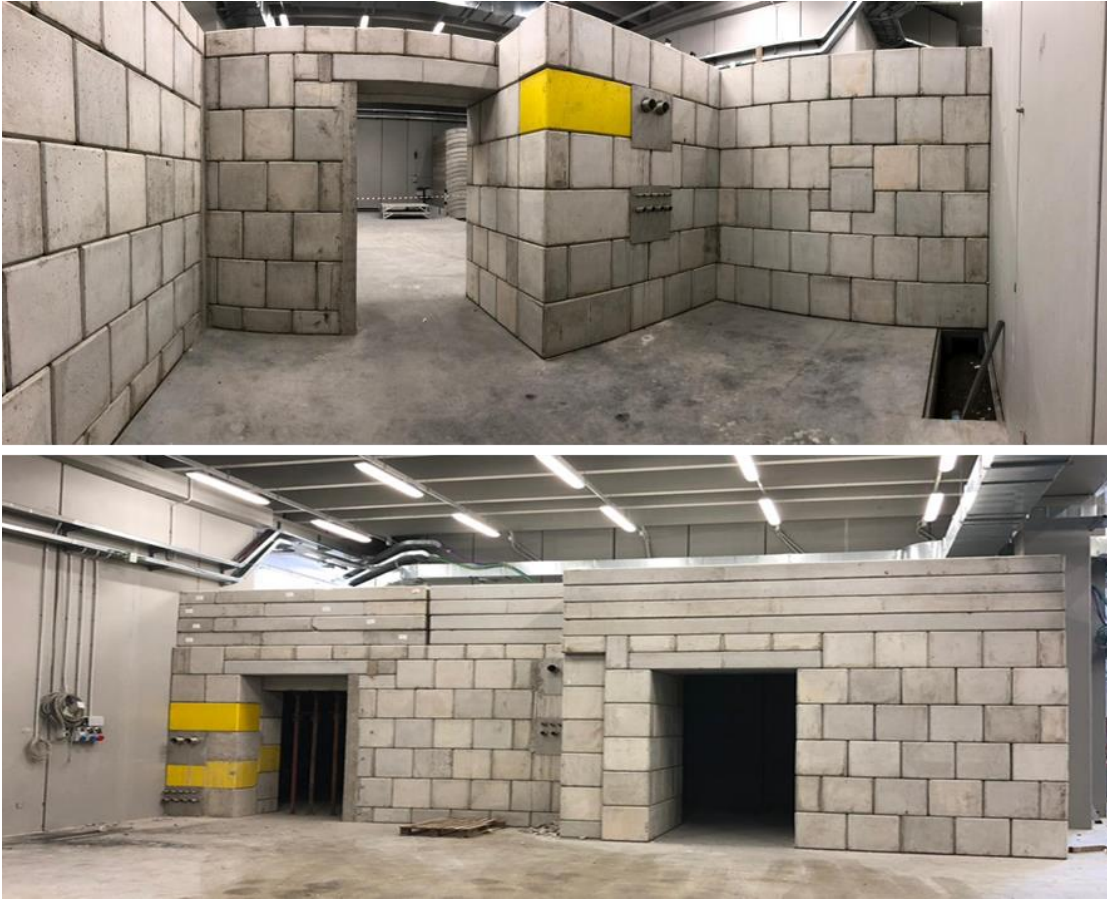
Figure 13: Civil works in progress for the A9c bunker previous the installation of the roof (may 2019) and completion of the whole structure (late summer 2019)
