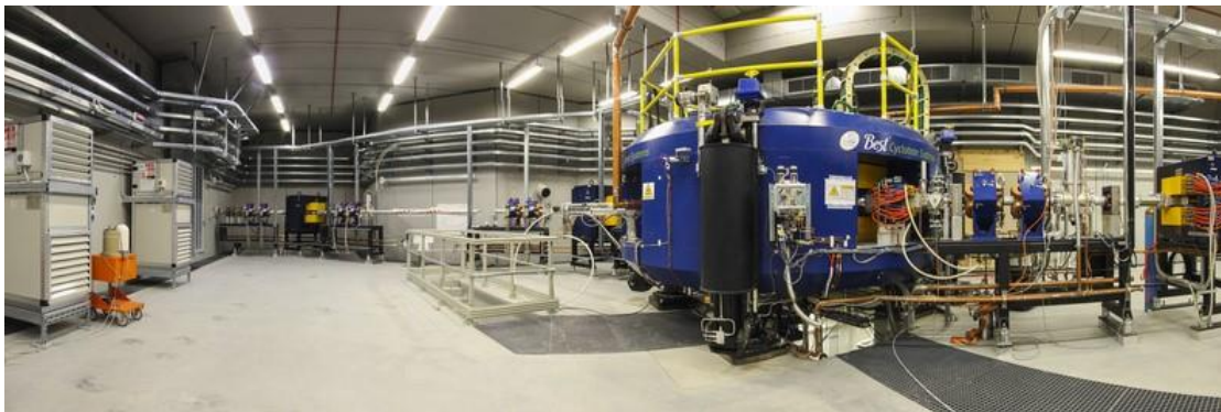
Figure 10: The new high-energy (35-70 MeV) and high-current (up to 750 \mu A) proton-beam cyclotron installed at INFN-LNL (Legnaro, Padua, Italy)
