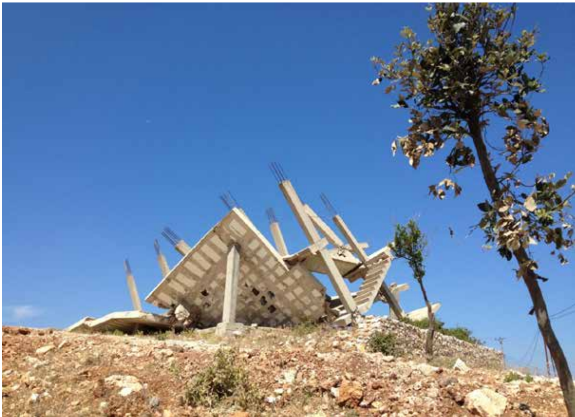
Figure 8-7. Demolished building in Ksamil (Albania). Source: author.
