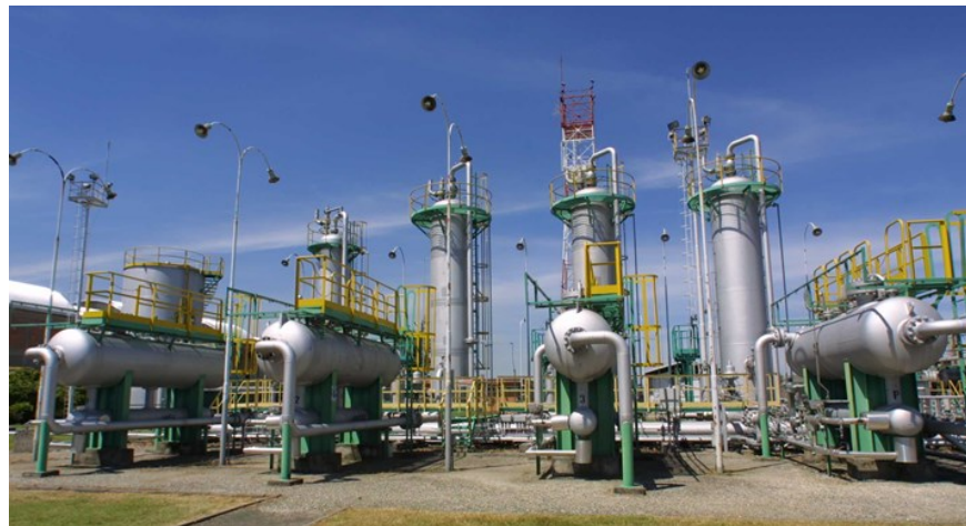
Fig.3 Natural Gas Storage Site, Minerbio, BO, Italy. ( www.stogit.com )
