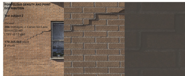
Figure 2. Quality check of the collected data, in this case the point cloud has a sufficient density and distribution of points to describe the elements that define the building
