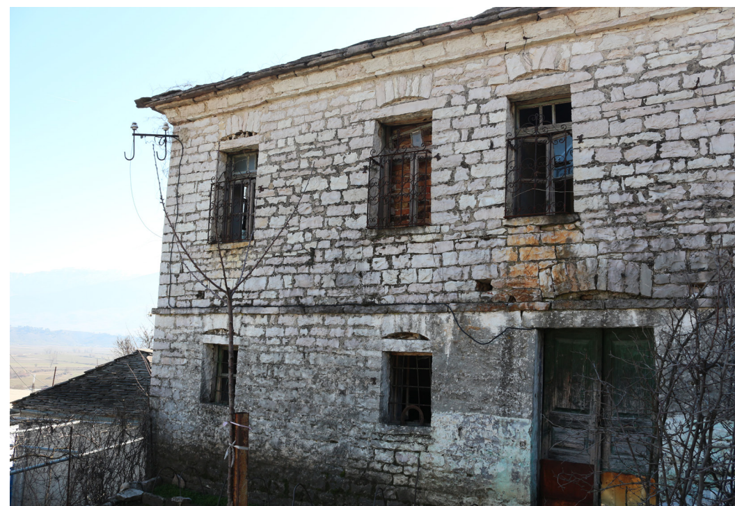
Fig. 1 / Traditional stone house on Dervician, the selected building (February 09, 2019) Source / the author
