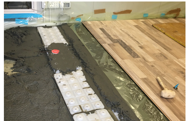
Fig. 3. RF installation with the positioning of the heat flux meter.
