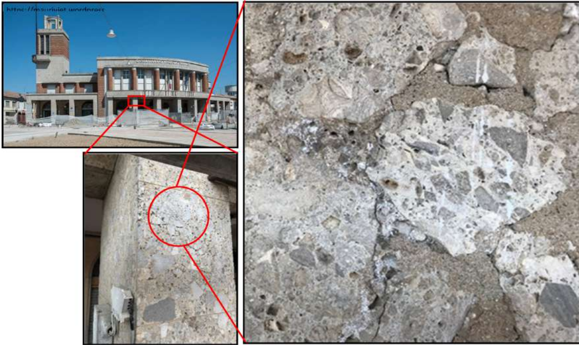
Figure 5. Concrete infilling mortar sample CO3. The Ex casa del Fascio building has been affected by damages caused by the earthquakes in May 2012, but before these events it was been subjected to restore operations not always made following the correct procedures for historical building.
