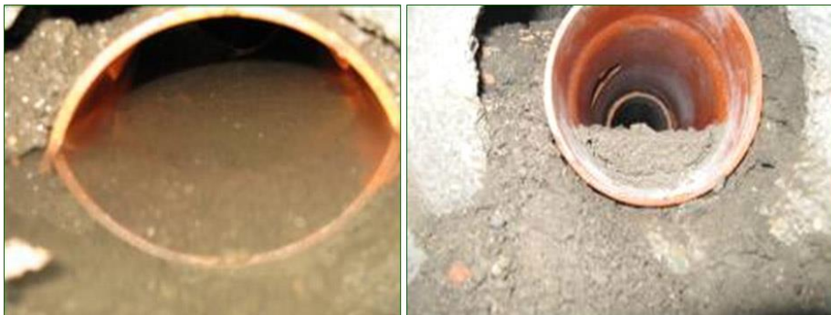
Fig. 9. Maintenance work are basic for efficiency of the plants, e.g. avoiding obstruction by water and ground.
