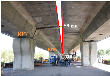
(a) View before installation and detail of the dislocation at joint “RP7”.
