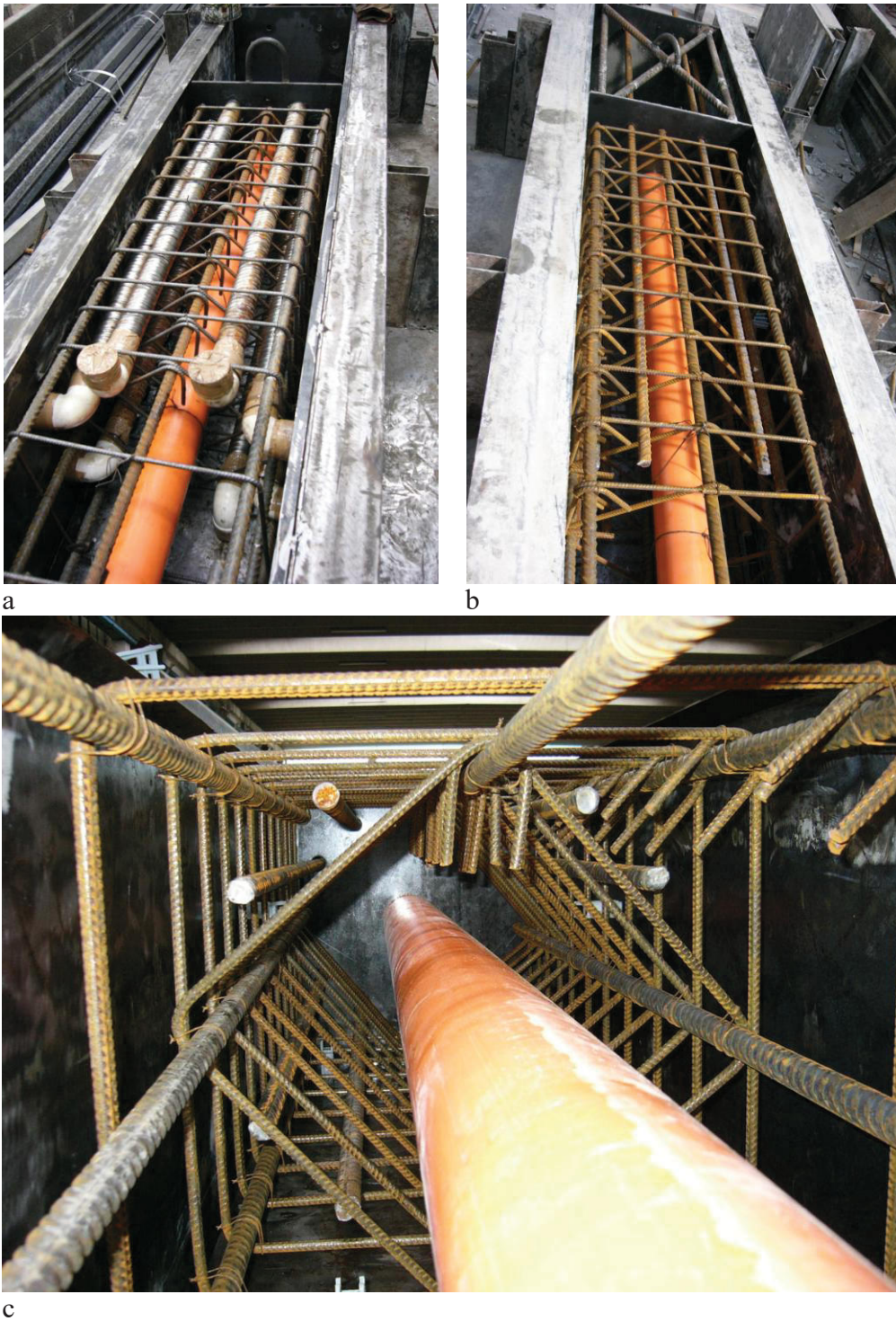
Fig. 2. Reinforcement cages for the precast column units: (a) stub columns A and (b) B; (c) detail view of stub column B showing the projecting bars and stirrups along the splice region.
