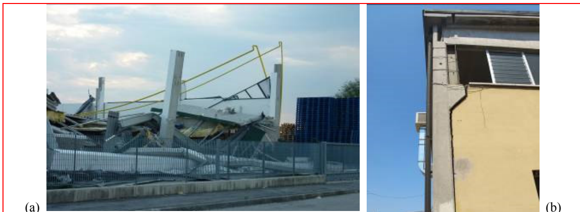
Fig. 6 Damages in precast RC columns: (a) extended building collapse caused by large column rotation due to foundation settlement; and (b) column rotation due to settlement at the foundation level, counteracted by the presence of an industrial concrete pavement
