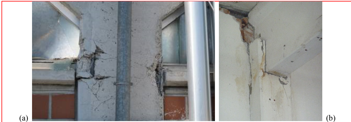
Fig. 5 Local damages in precast RC columns: (a) failure mechanism due to interaction with masonry infills; and (b) damage of the upper fork of a column due to flexural-torsional displacements of the precast beam
