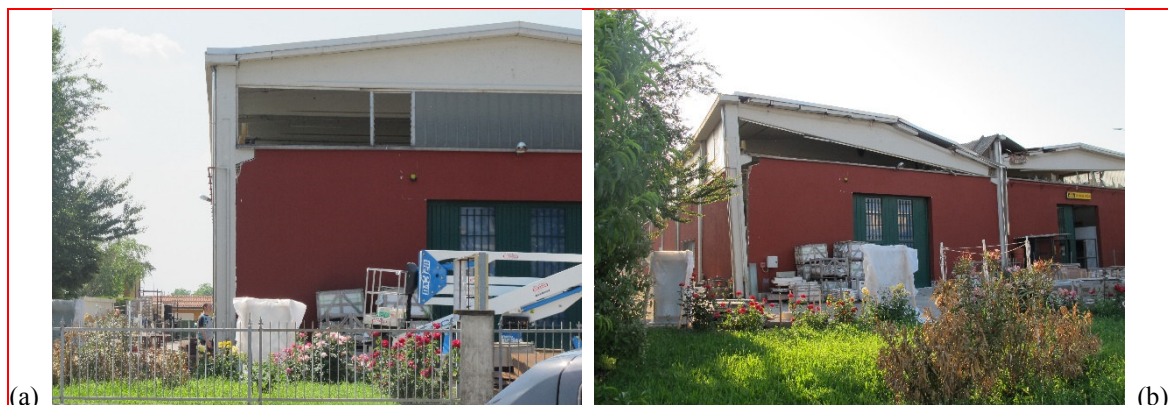
Fig. 7 Industrial building in San Giacomo Roncole (Mirandola, MO): (a) the building after May 20 th earthquake, and (b) after May 29 th earthquake
