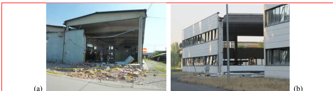
Fig. 3 Collapse of (a) a masonry curtain wall not restrained by the RC structure; and of (b) RC cladding panels due to failure of the steel channel profiles supporting them
