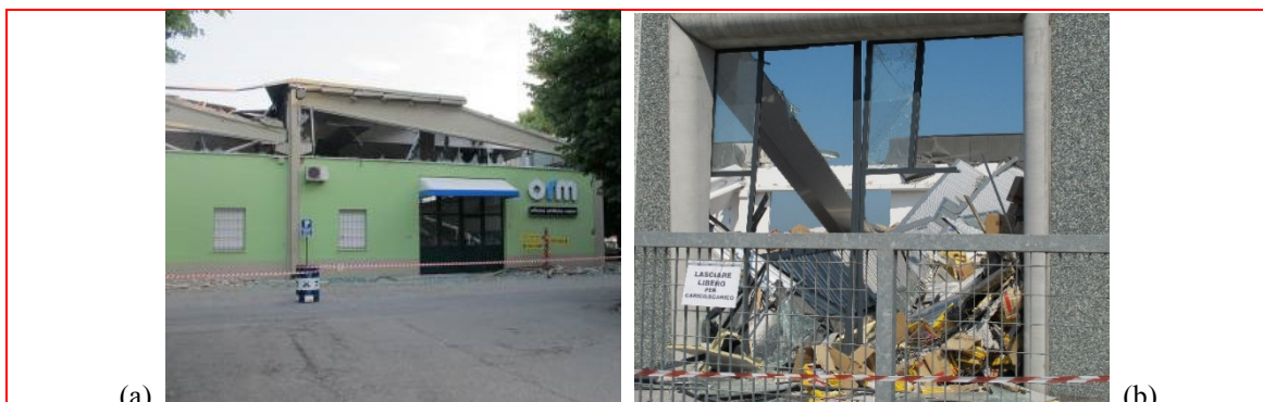
Fig. 2 Roof collapses in precast buildings: (a) partial collapse due to interaction with masonry curtain walls; and (b) extended collapse in a modern prefabricated building
