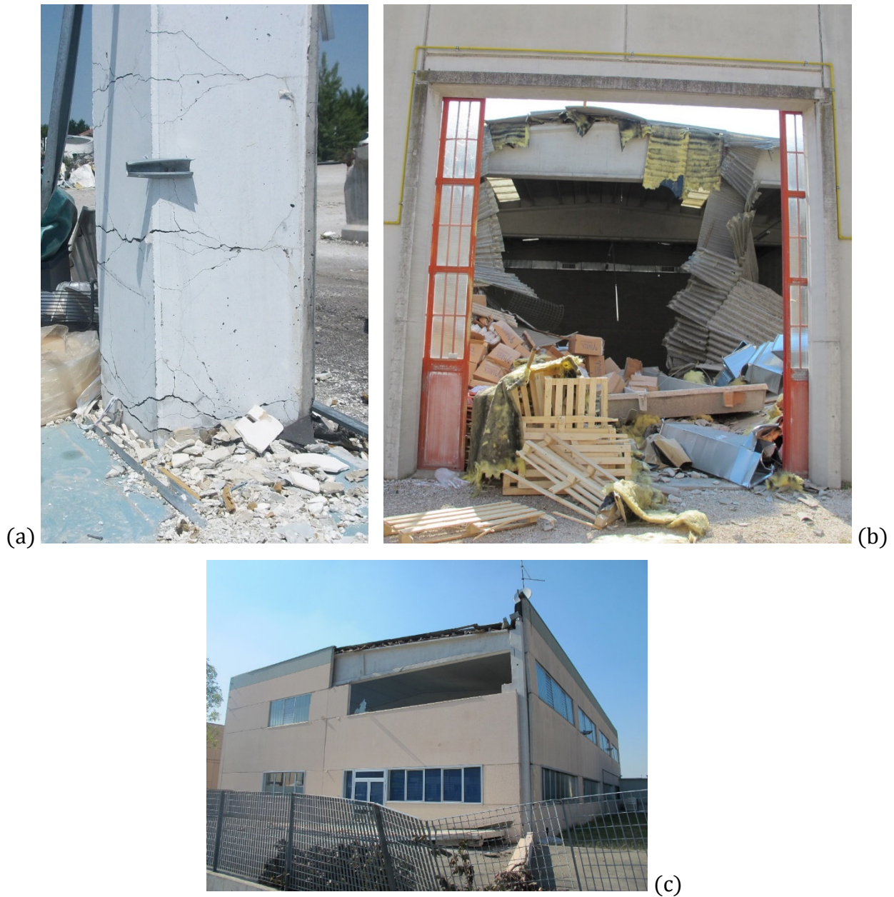
Fig. 2. Typical damage observed in precast buildings struck by the Emilia earthquakes: (a) plastic hinge at the base of a column; (b) loss-of-support of a simply-supported roof slab from main girders; and (c) out-of-plane overturning of RC cladding panels.
