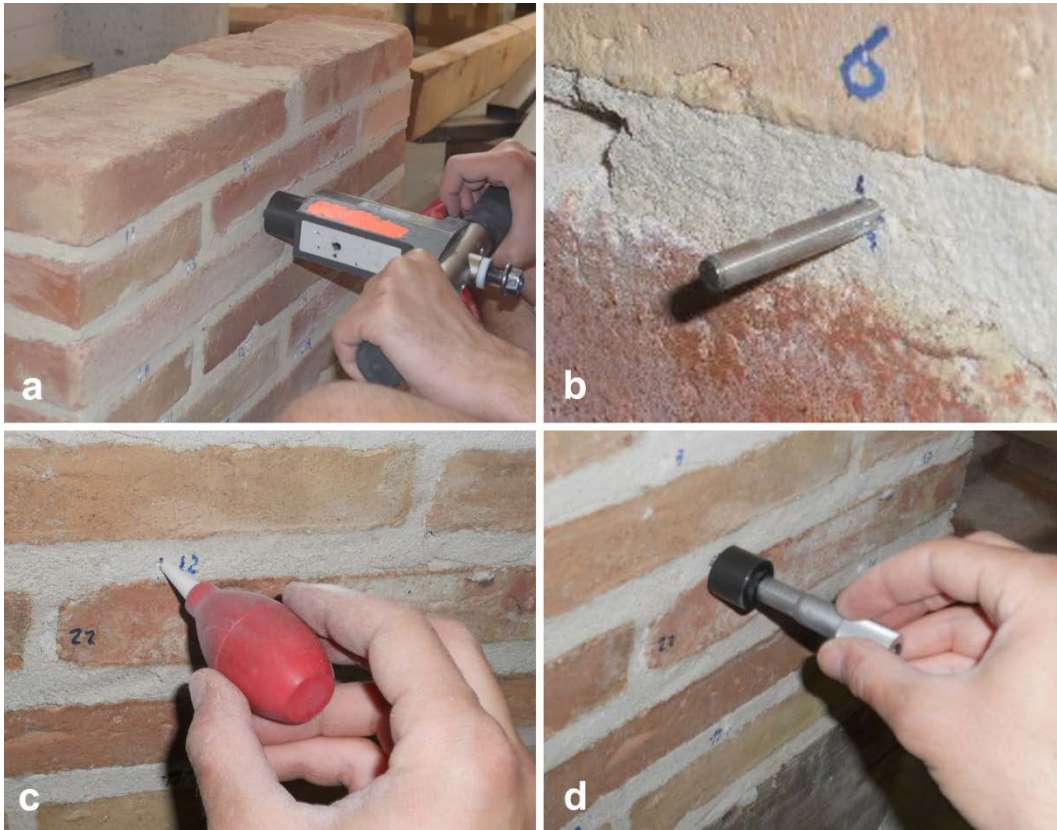
Figure 8 – Operation of the Windsor pin penetration test: instrument for pin insertion (a), pin penetrated into the mortar joint (b), cleaning of the indentation produced by the pin (c) and micrometer for depth measurement (d).
