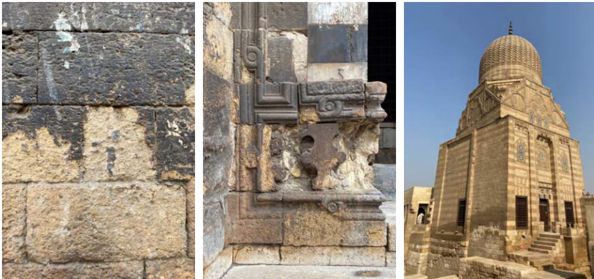
Figure 1. Common evidence of limestone decay in Medieval buildings in Cairo.
