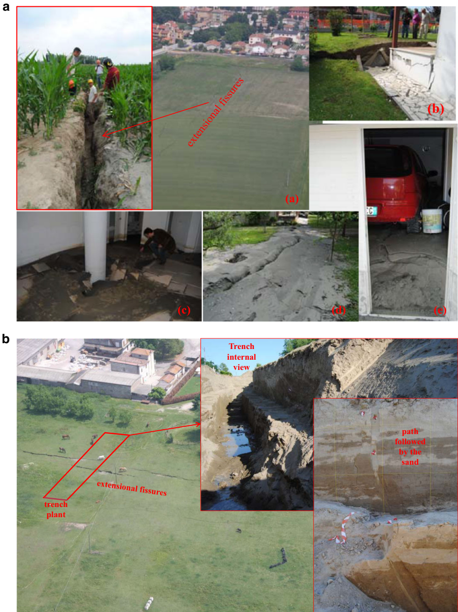
Fig. 3 a Liquefaction effects and b 6 m deep exploratory trench
