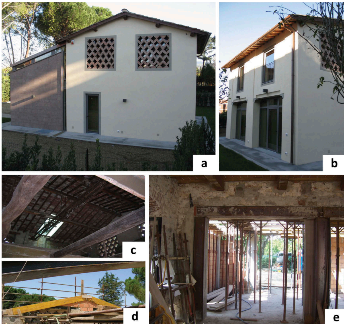
Figure 3. Example of widespread local interventions on a former rural building (hayloft and agricultural machines storage), subject to adaptive reuse as an office building in a suburb of Florence, Italy. (a–b) Post-operam results; (c) Roof timber structure (ante-operam); (d) activities on roof structure; and (e) metal frames recovering stiffness of demolished masonry panels.
