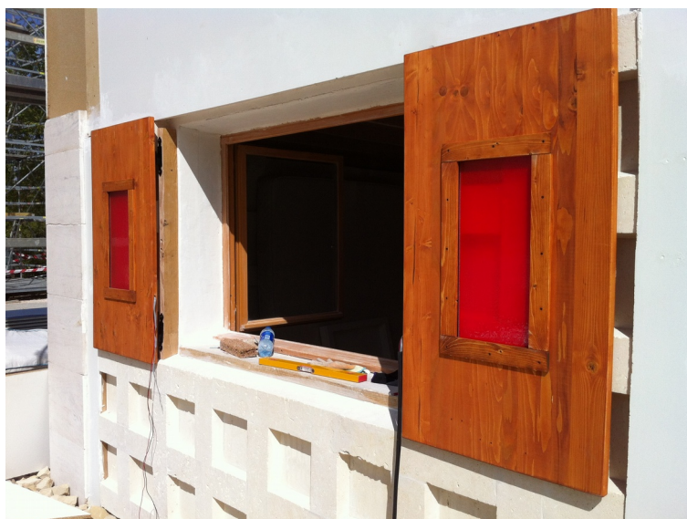
Fig. 6.1.1: The solar shutters installed on the Astonyshine house at SDE2012, the photo is taken during the construction of the house
