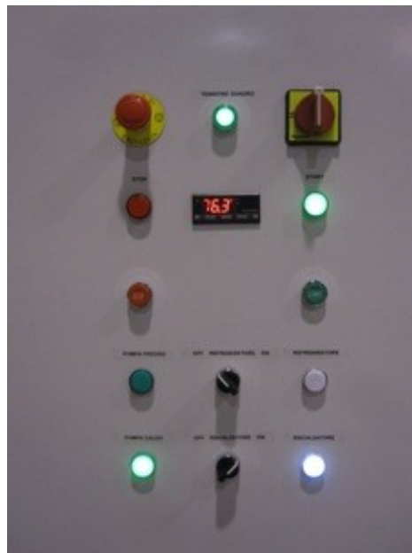
Figure 3.3 – Digital image of the electric board
