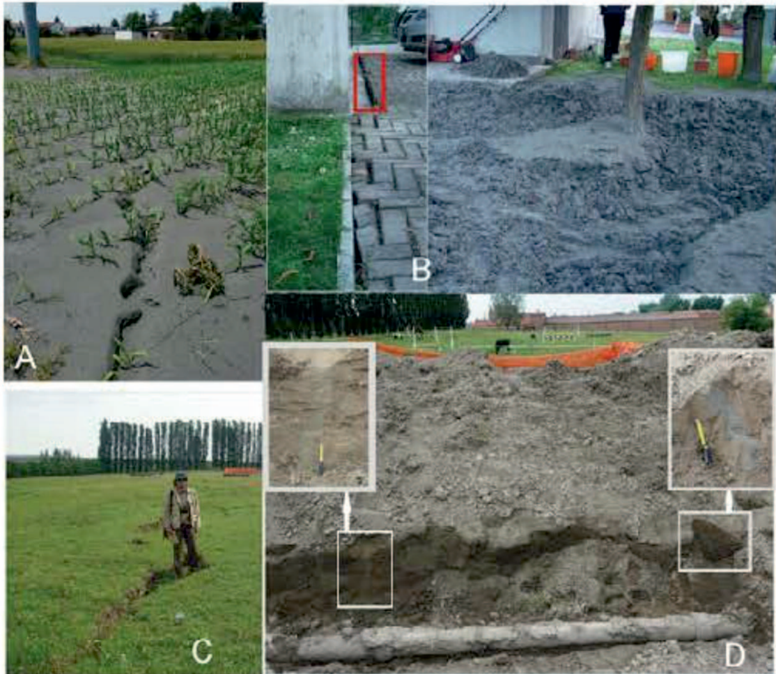
Figure 2.8: A) Vent fractures with ejected sandy material. B) Sandy material covering the courtyard of a settled and shifted house. C) Surface ruptures. D) Evidence of a penetration of a clayey cap layer by a sandy material (from Caputo and Papathanassiou, 2012) .
