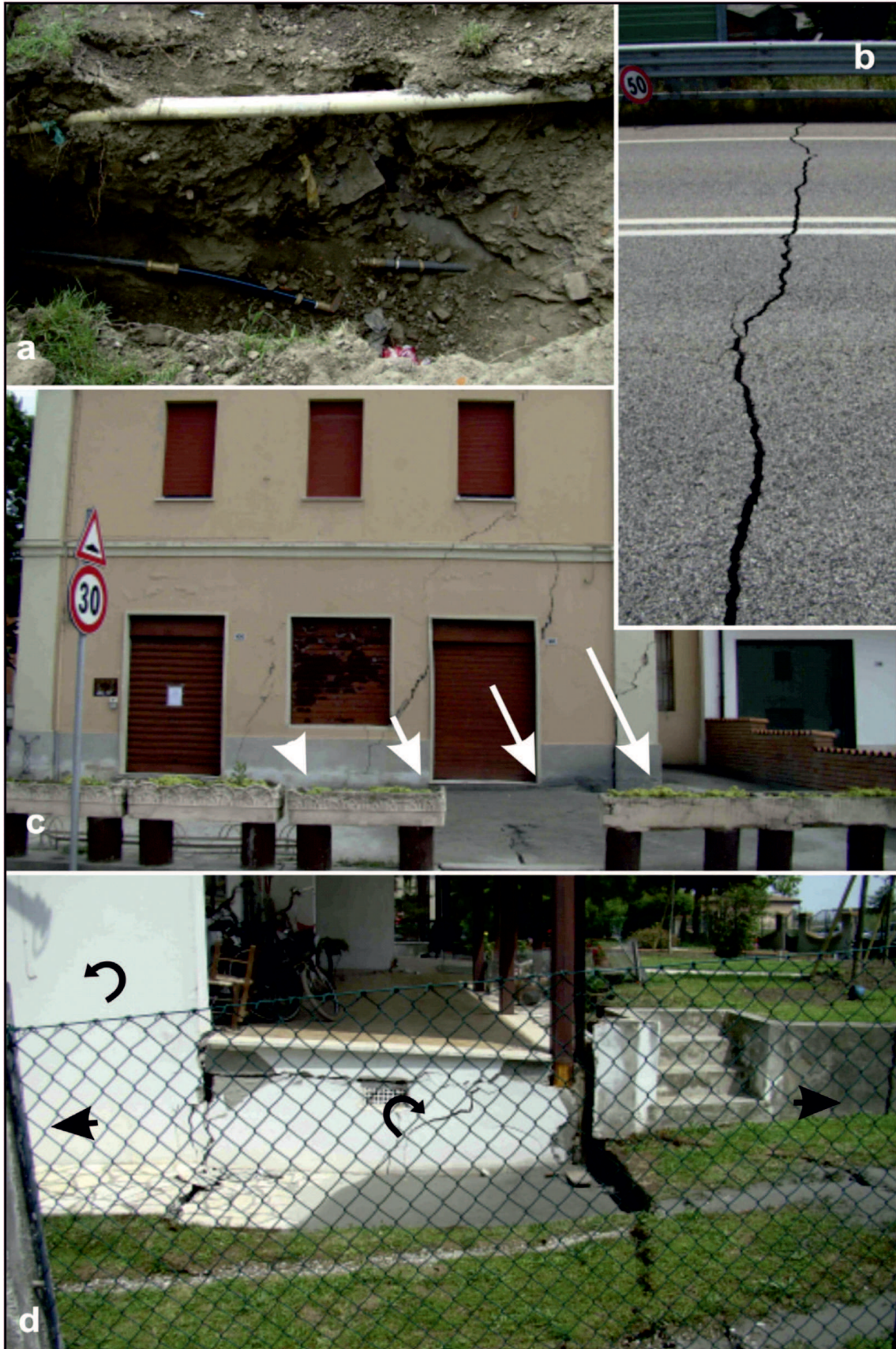
Figure 6.24: Examples of damages produced by the May 20, 2012 earthquake. a) Broken pipelines. b) Paved roads. c) Buildings with cracking due to differential settlement. d) Lateral spreading (from Papathanassiou et al. , 2015).
