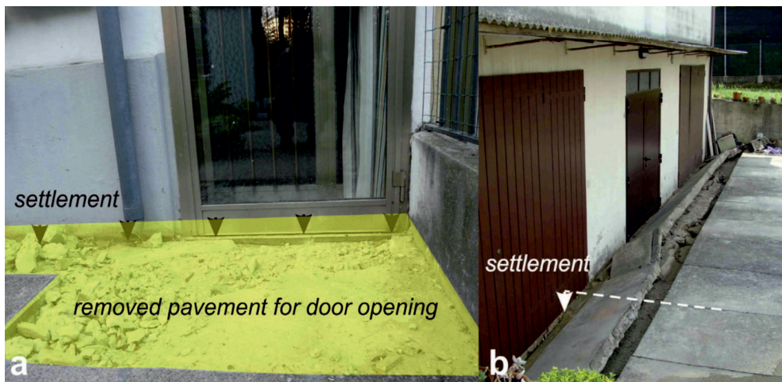
Figure 6.26: Examples of ground loss due to liquefaction and consequent settlement of the buildings (from Papathanassiou et al. , 2015).
