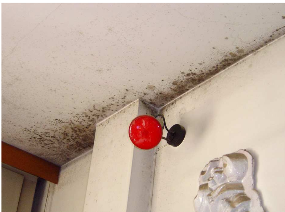
Figure 6.9 – Ceiling's mould in the apartment
