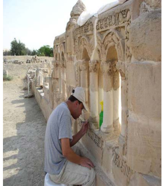
Figure 4.21: Restoration projector of the sandstone of Hisham's Palace
