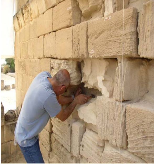
Figure 4.20: Restoration projector of the sandstone of Hisham's Palace
