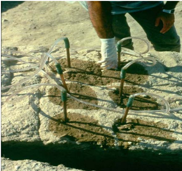
Figure 4.16: Using ethyl-silicates and Primal techniques to consolidate ancient mud-brick walls in Tell es-Sultan. (Source: MoTA Archive)
