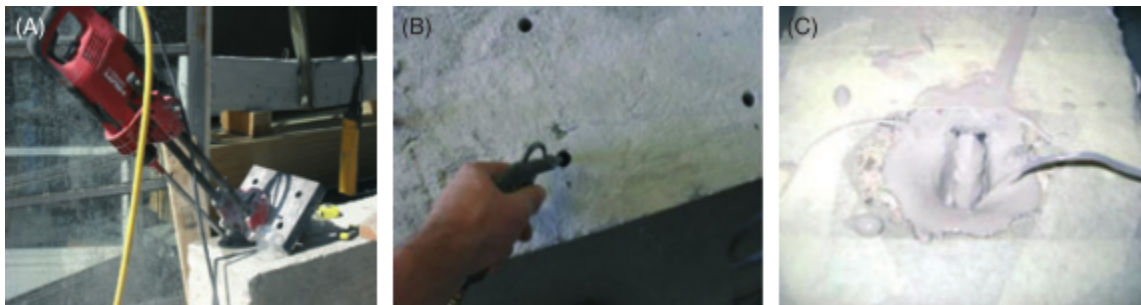
Fig. 2.34 Embedded Through-Section (ETS) strengthening technique as reported in (Barros and Dalfré 2012): (a) drilling of the holes, (b) cleaning of the holes with compressed air, (c) hole filled with adhesive and ETS strengthening bar.
