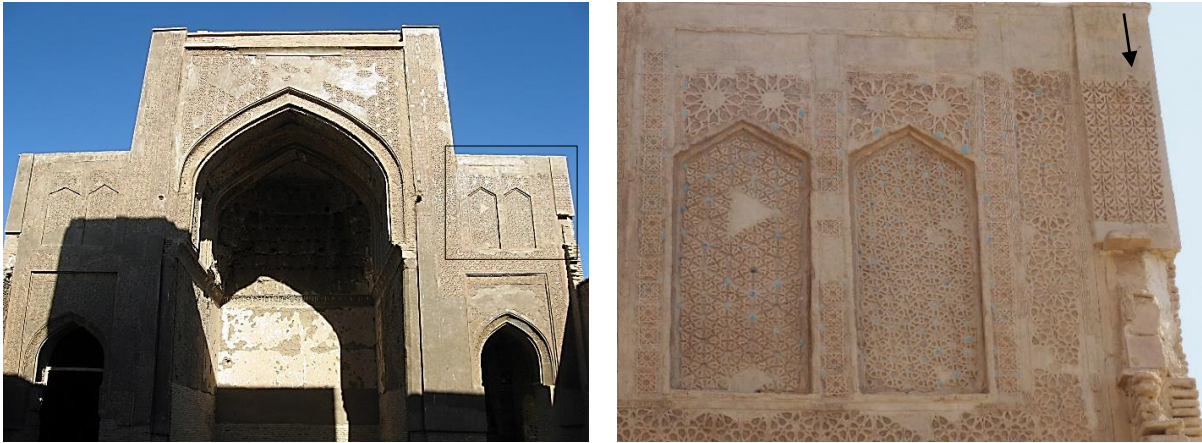
Figure 2.27. The north-eastern façade (left) and the details of its decoration (right) at the Farumad mosque
