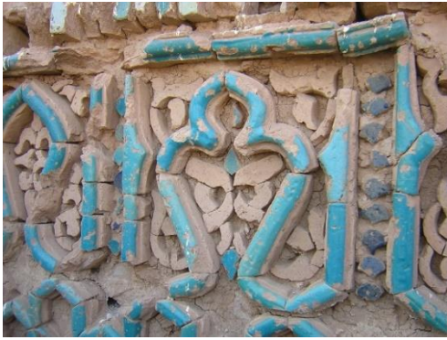
Figure 2.18. The alternating keyhole and segmented arches in the upper zone of the inscription on the back wall of the qibla iwan
