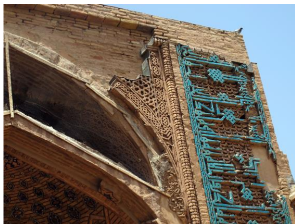
Figure 1.9. Eastern portal of the Masjed-e Jāme'-e Herat showing Ghurid ornaments (brickwork and glazed inscription) and Timurid alterations.
