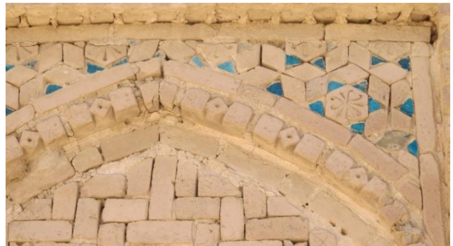
Figure 2.5. The lozenge and hexagonal bricks and the inset triangular glazed ornaments at spandrel of the blind arch (the eastern façade of the north iwan)
