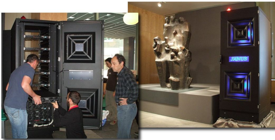
Figure 3.1 – The Janus rack during the installation for the unveiling in Zaragoza in Spring 2008.
