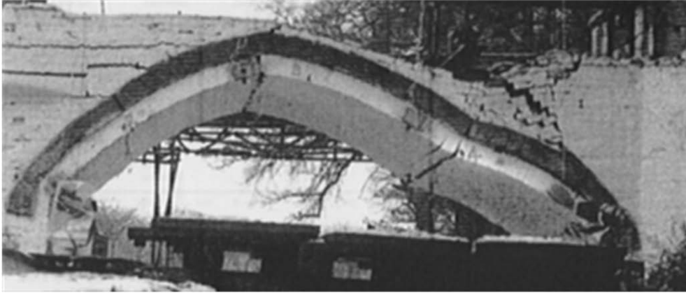
Fig. 8: Collapse of Prestwood Bridge [41].
