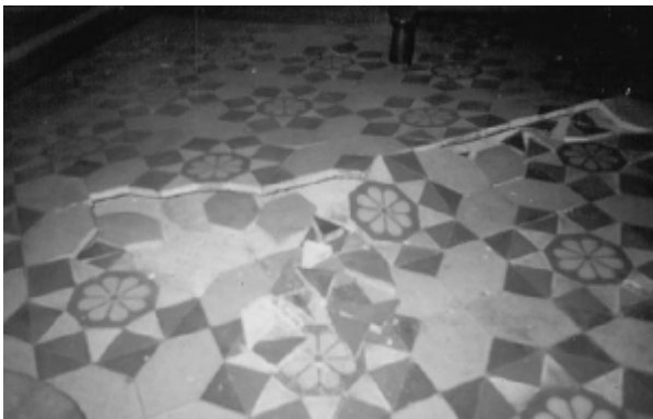
Figure 4. Complete collapse of a tiled floor after severe water penetration (Oddy & Linstrum, 2005)
