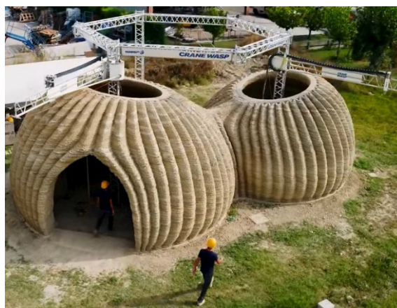
Fig. 5. WASP (Italy’s pioneering specialists in 3D printing) has completed the printing phase of the TECLA supporting structure, the first and unique fully 3D printed construction based on natural materials and made with multiple 3D printers operating at the same time. The innovative habitat model engineered by WASP and designed by MCA - Mario Cucinella Architects was conceived as a new circular model of housing entirely created with reusable and recyclable materials, sourced from local soil, carbon-neutral and adaptable to any climate and context. Source: Alfredo Milano, CC BY 2.5 < https://creativecommons.org/licenses/by/2.5 >, via Wikimedia Commons
