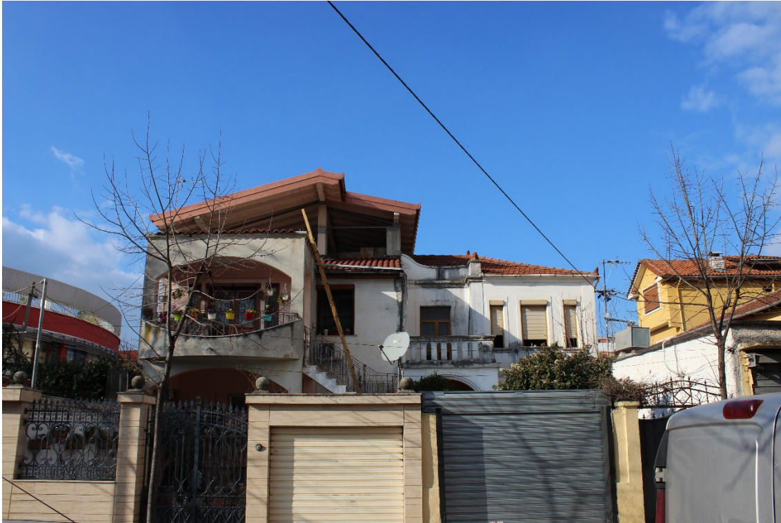
Figure 46: The villa was divided into two symmetrical parts, as two brothers inherited the villa. Source: Author, 2020
