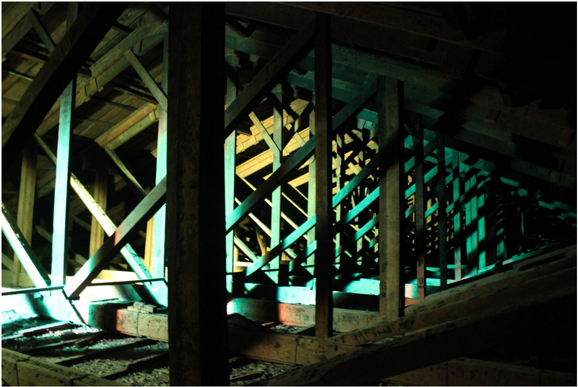
Photography of the inside the space of the roof of the theatre. Source: Author, 2019
