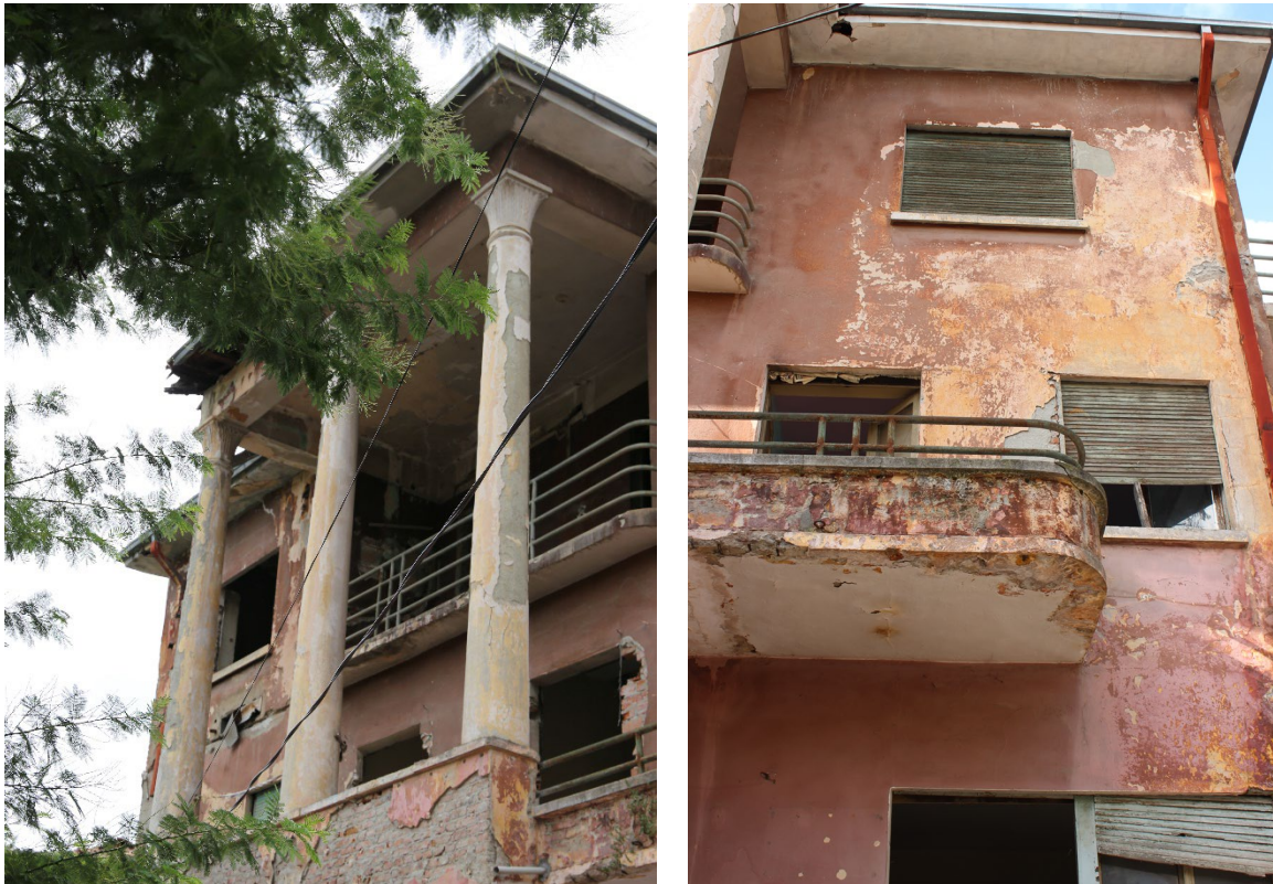
Figure 37: Former Radio Tirana building left in decay; Source: Author, 2020
