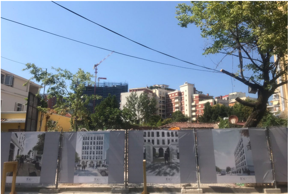
Figure 44: Villa Destil After the destruction, the fenced plot is ready to start building works. Source: Author, 2020
