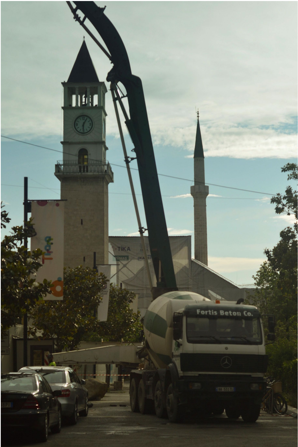
Photography of the construction site next to the clock tower of Tirana. Photo courtesy Artan Rama, 2020
