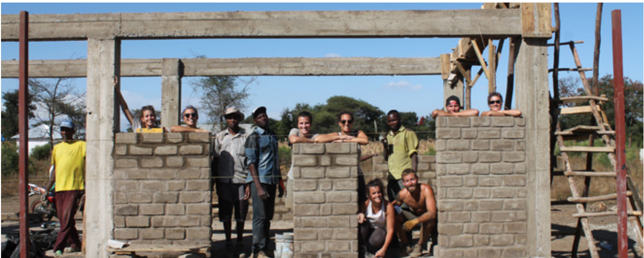
7.33 Team working on the construction of the closing CSEB wall after completion of the concrete structure. Source: Own picture.
