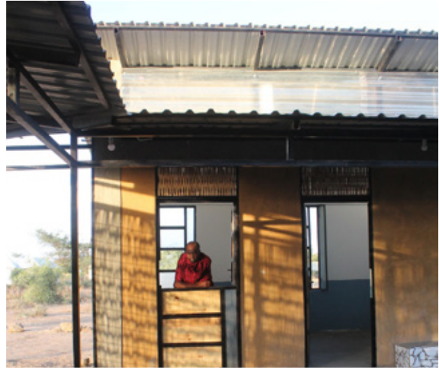
7.39 Reception room and observation room. To note the timber of the doors re-used from casting. Source: Own picture
