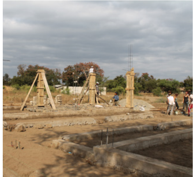
7.25 Finished over foundations and casting of the concrete pillars of block 1. Source: Own picture
