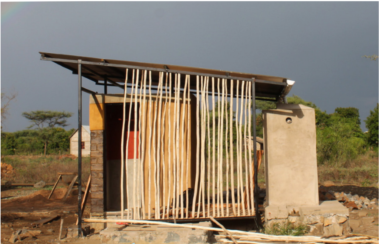
7.14 Dispensary's toilet block from the front and right side. See the water tank which collects rainwater. Source: Own picture
