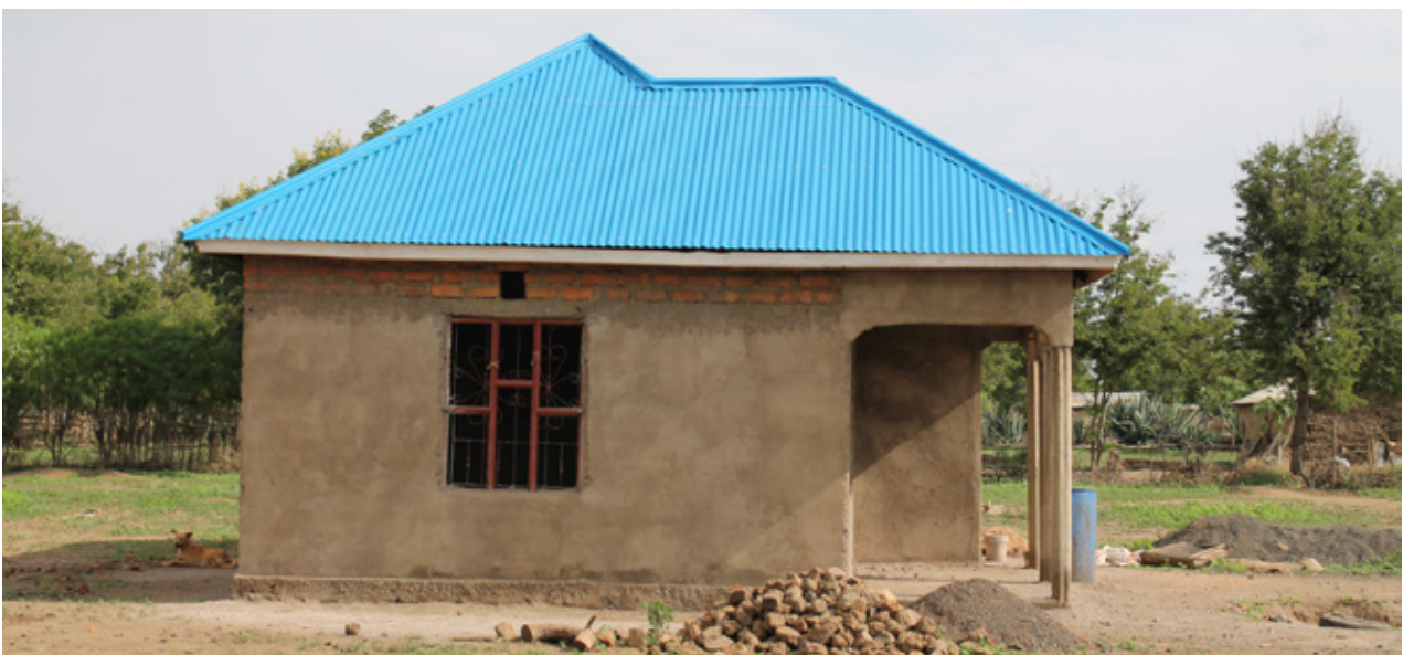
13.10 House under construction in Maji Moto, built with fired bricks and plastered with cement. This is the current trend style of house raising in the area. Source: Own picture
