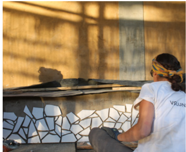
7.41 A volunteer working on the finishing detail of the bench, using re-used broken tiles. Source: Own picture
