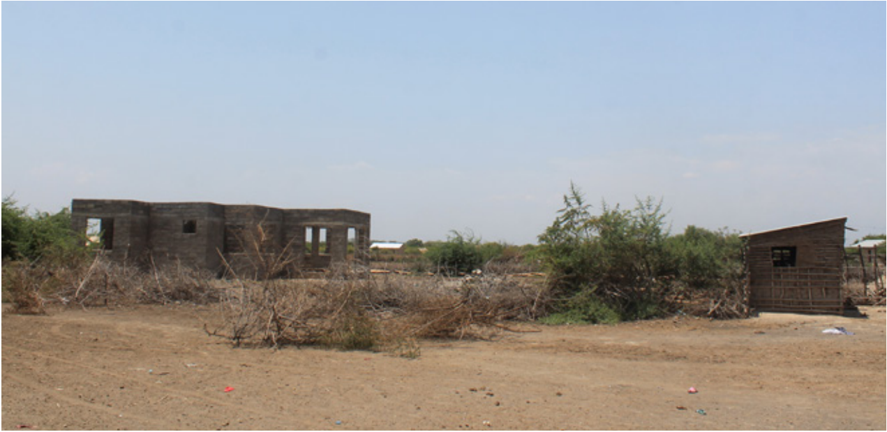
12.12 Within Jesse's plot, the house on the left side is being built with concrete blocks, where the family will move after completion. Source: Own picture
