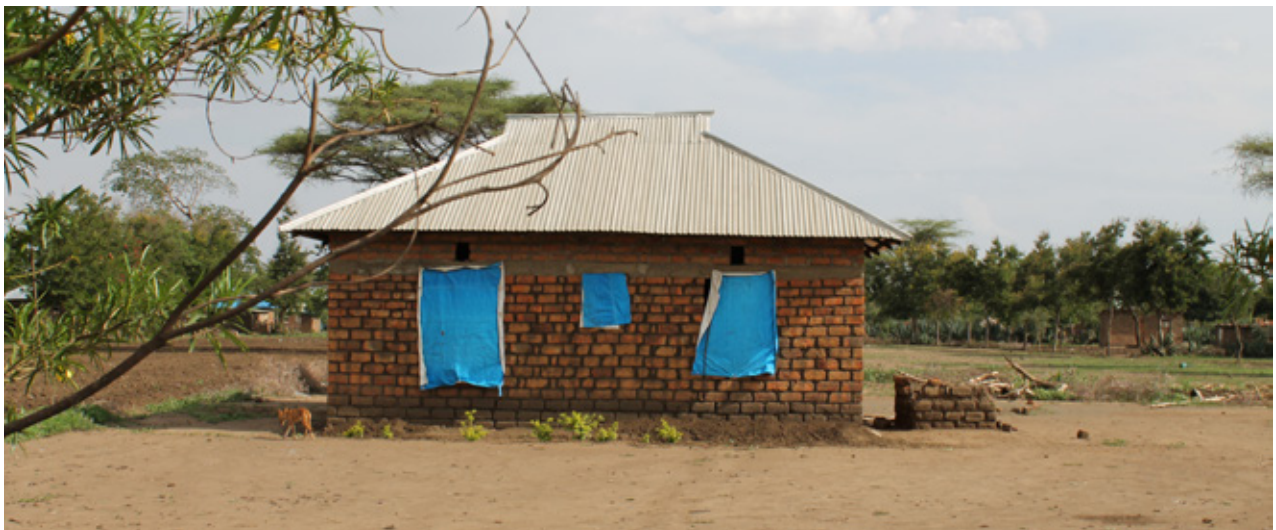
3.19 Fired brick house under construction in a Maasai area close to Arusha. Source: Own picture
