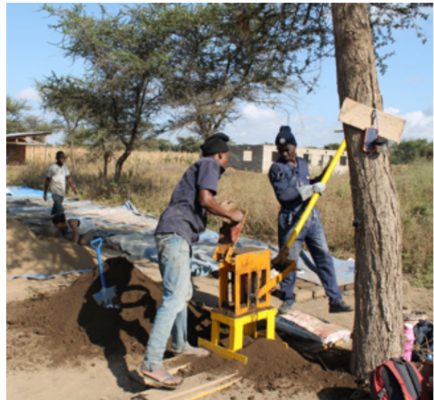
7.27 Construction workers producing CSEB on the site of the dispensary. Source: Own picture
