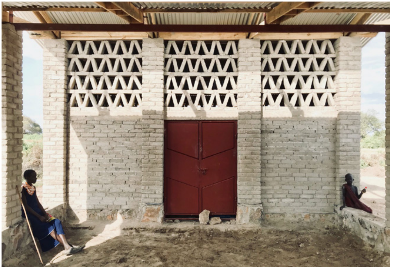
8.7 Detail of the bricks' lattice work that ventilates and illuminates the indoor shop. Picture before completing the floor. Source: C-re-aid website
