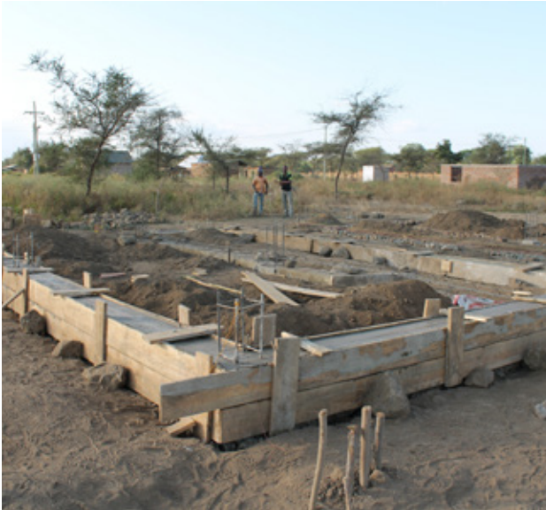
7.24 Form works containing the concrete structure of the over foundation. Source: Own picture
