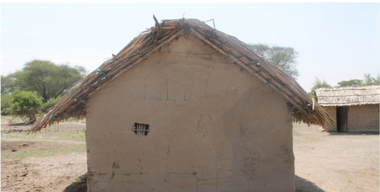
13.12 Typical earth house in Mikocheni, constructed with the wattle and daub technique. Little cracks are visible within the house walls. Source: Own picture
