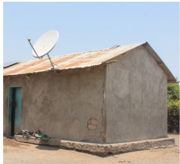
13.4 Yesse's house in Mikocheni, with visible cement plaster that is peeling off from the adobe bricks' wall. Source: Own picture
