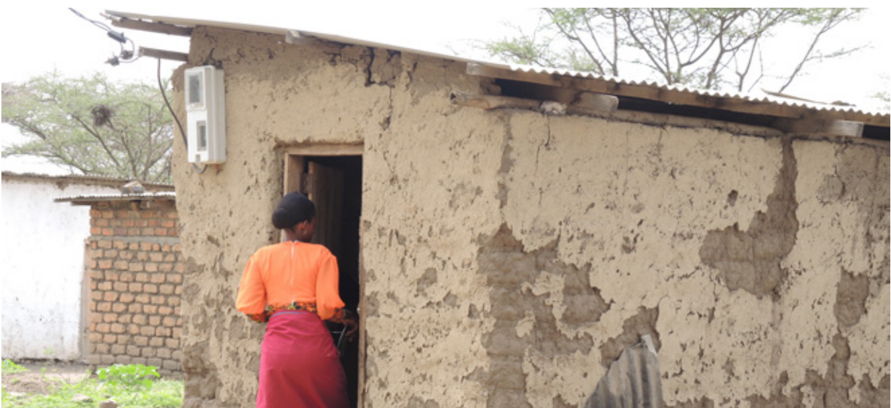
14.5 A woman enters a kitchen in Maji Moto built with adobe bricks. The surface of the walls is visibly deteriorated. Source: Own picture
