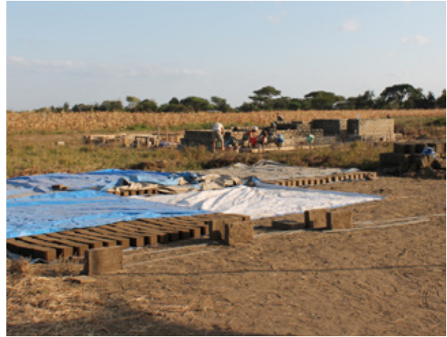
6.18 CSEB drying on construction site after production and ready to be cured before piling after 2 days. Source: own picture
