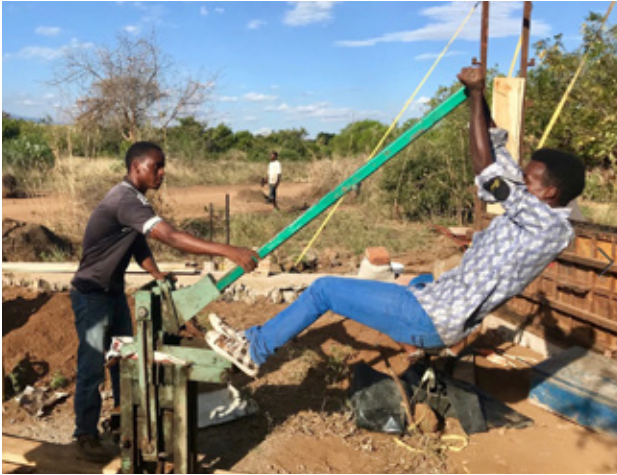
6.17 Skilled workers using the compressing machine to produce CSEB on site. Source: Own picture
