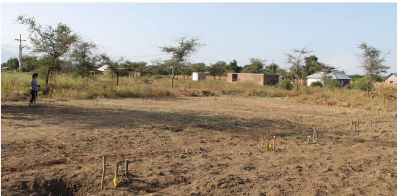
7.23 Construction site after cleaning and measuring the foundations before digging. Source: Own picture
