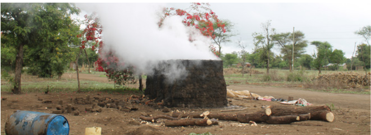
6.7 Hand-made fired bricks' kiln baking for the second day in Maji Moto. Source: Own picture
