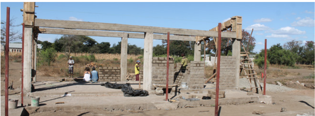
7.28 Dispensary's block one with concrete structure completed, both columns and beams. Source: own picture
