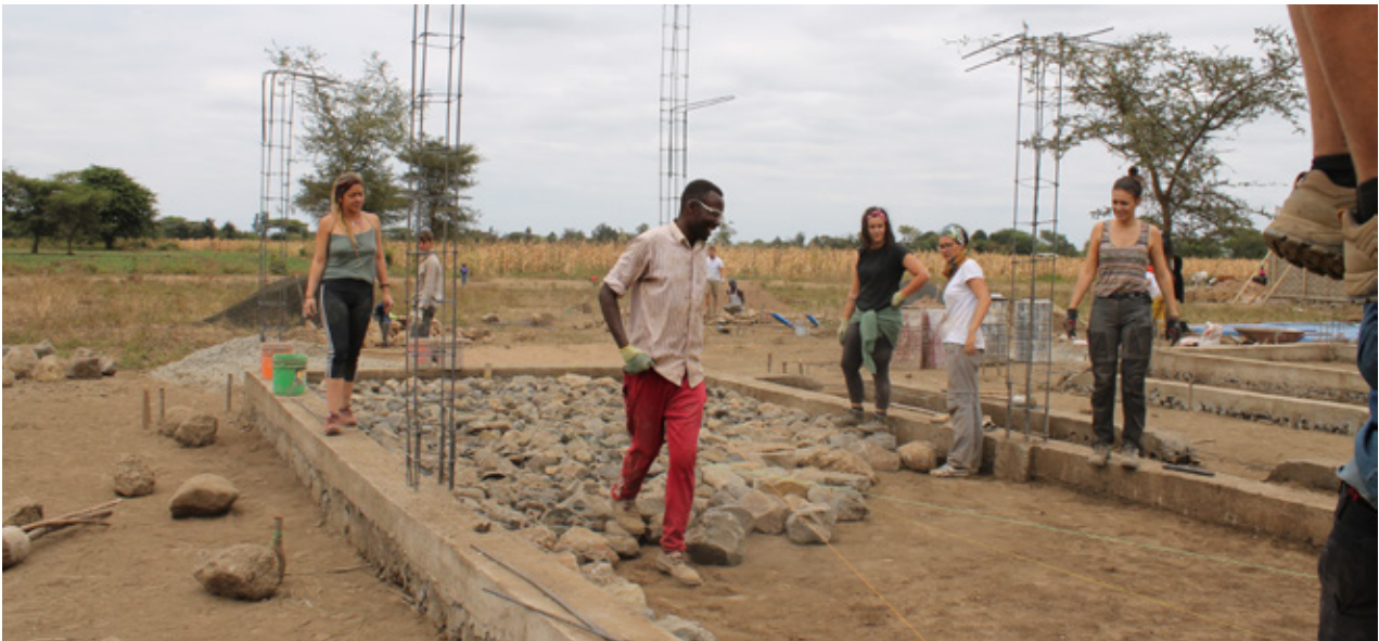
7.31 Team working on the filling of the floor slab with local stones, before pouring concrete on block 2. Source: Own picture
