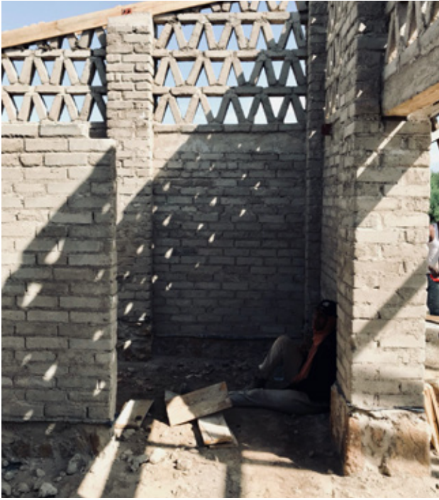
8.14 The shop under construction that highlights the CSEB lattice work. Source: C-re-aid website
