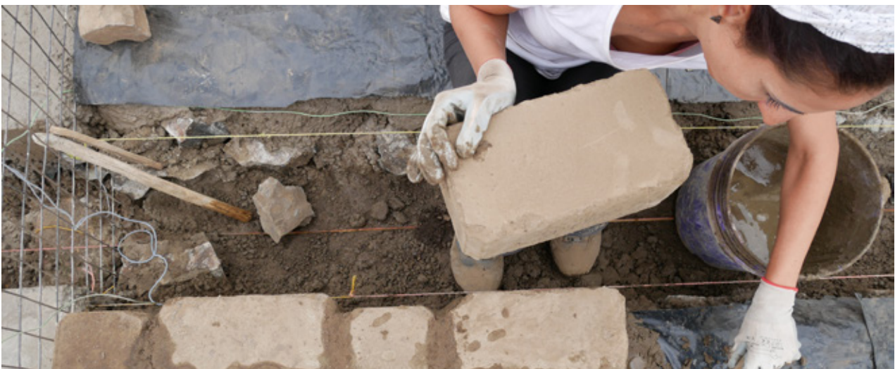
7.34 Volunteer working on the CSEB construction of the toilet's water tank. Source: Own picture.
