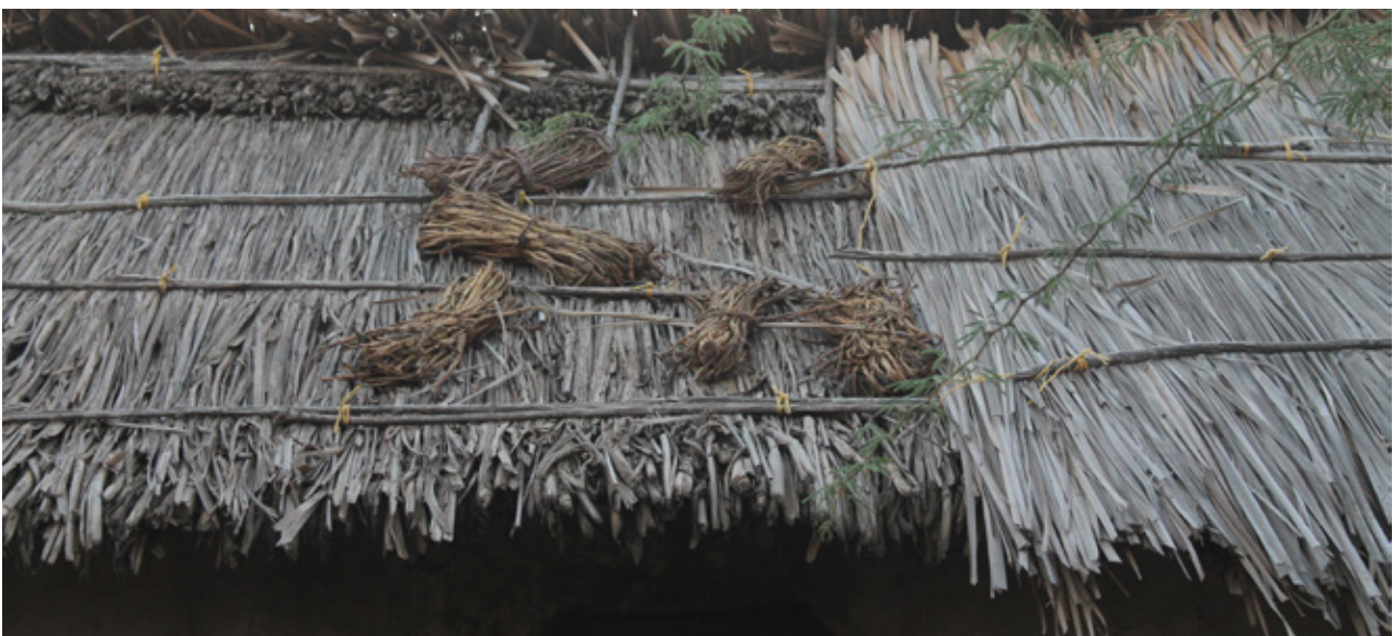
14.4 New layer of thatch is being added to a roof in Mikocheni, tiding them up with ropes and further securing the roof with wooden sticks. Source: Own picture
