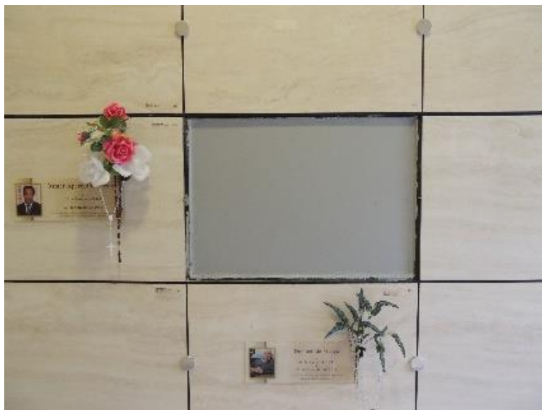
Figure 14 - Structure of the niches of the Necrópole Ecumênica Vertical Universal (Curitiba, Brazil) to avoid contamination from the decomposition process in the indoor environment.
