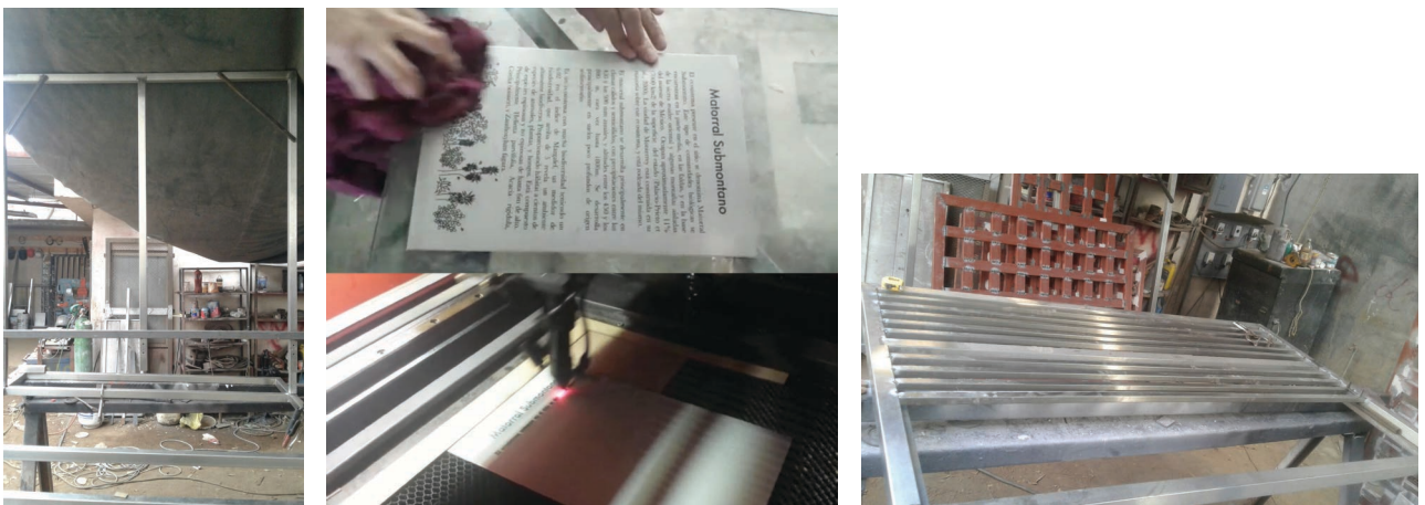
Metal components of the landscape installations under fabrication, February 2017. (photos: Jaime Islas)
