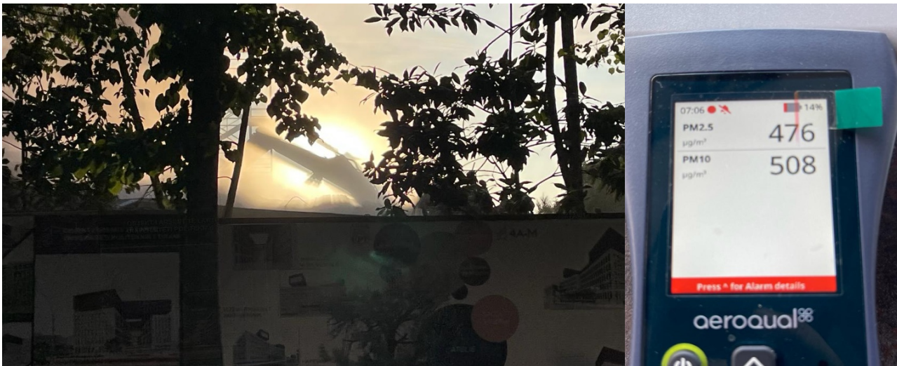
Figure 18: PM concentration exceeding 10 times the standard due to demolition of the Faculty of Civil Engineering
