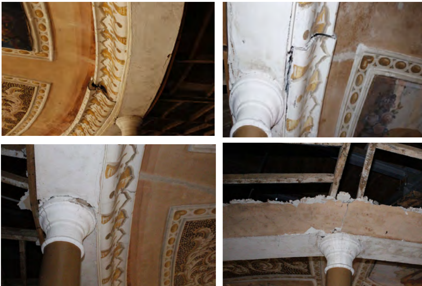
Detailed views of the damage found across the gallery border
