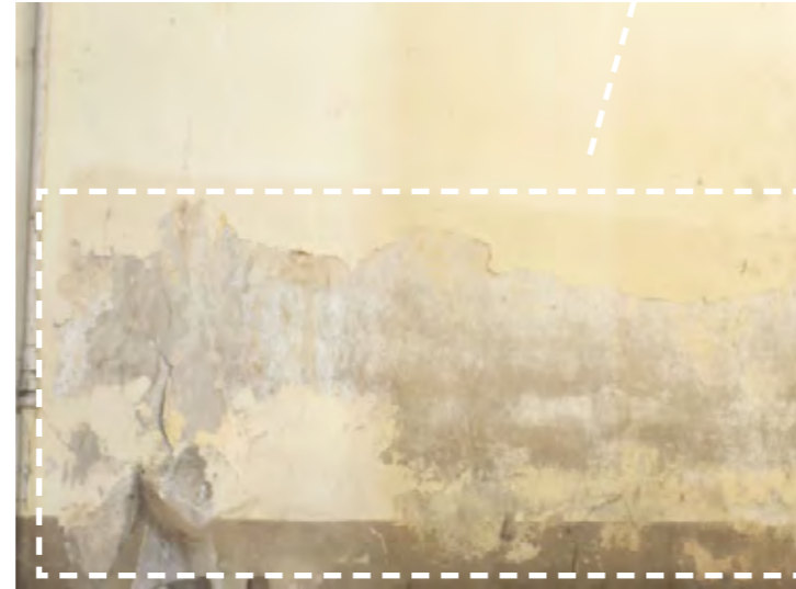
macro detail of the plaster detachment partially visible in photo 4
