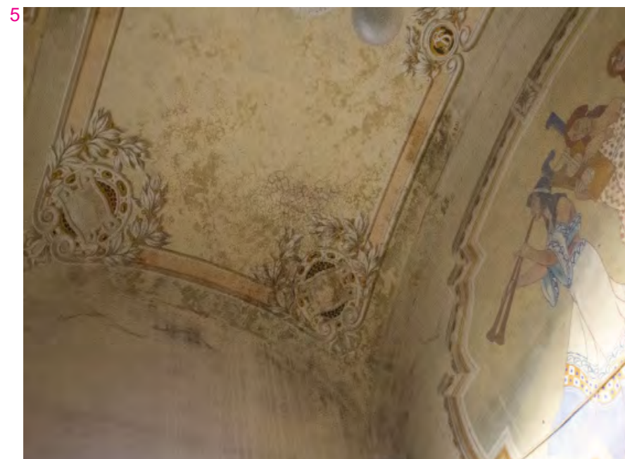
3-4-5 staining: localised colour variation of the plaster surface
