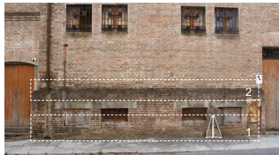
1-rise; biological colonisation 2-dripping; biological patina: the phenomenon is linked to inadequate water disposal..
