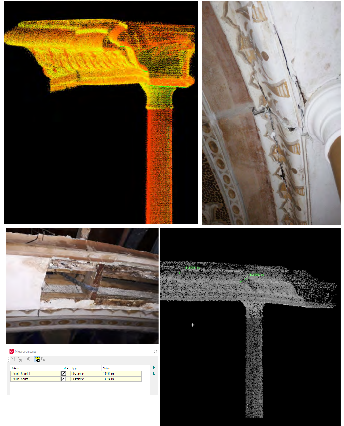
Detailed views of the damage found across the gallery border
