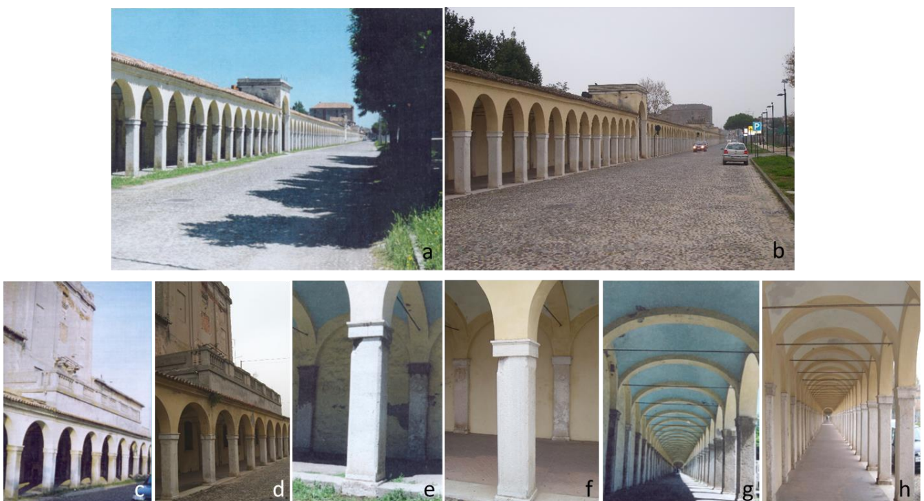
Figure 2. Pictures of different part of the Loggiato dei Cappuccini: (a,c,e,g), before the 2009 restorations (images from the municipality of Comacchio); (b,d,f,h), the corresponding current state condition.
