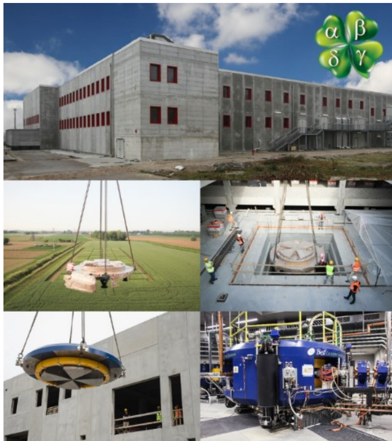
Figure 10 Pictures of different moments of SPES realization: from the top SPES building and cyclotron installation phases (LNL-INFN, SPES facility).
