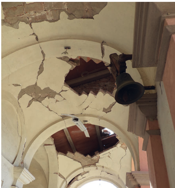
Fig.33. Concordia Sulla Secchia Cemetery (Modena crater area). Vaults without ties damaged by the earthquake.
