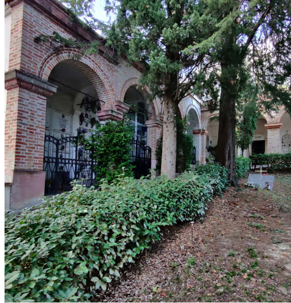
Fig.4. Cemetery of Airo (Marche region) Columbaria in a slope configuration. Ph Arch. Marta Zannotti
