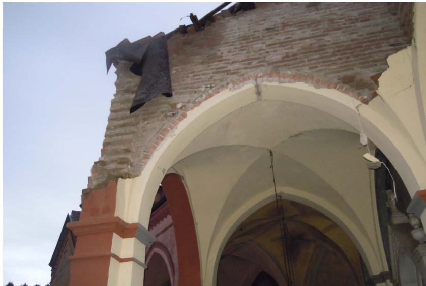
Fig.8. Bondeno cemetery (Ferrara crater area): building collapse at the growing interface. It should be noted the brick disposition that emphasise an addition.
