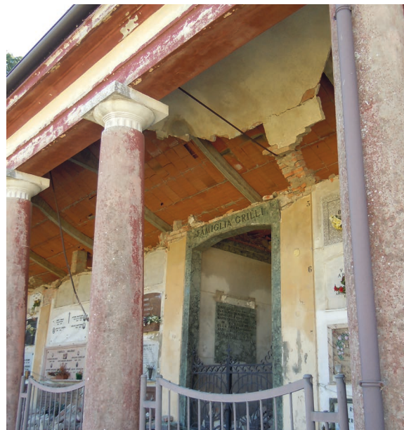
Fig.34. Mirandola Cemetery. (Modena crater area). The vaults ties were ineffective as they were anchored to small walls on the side of the columbarium.
