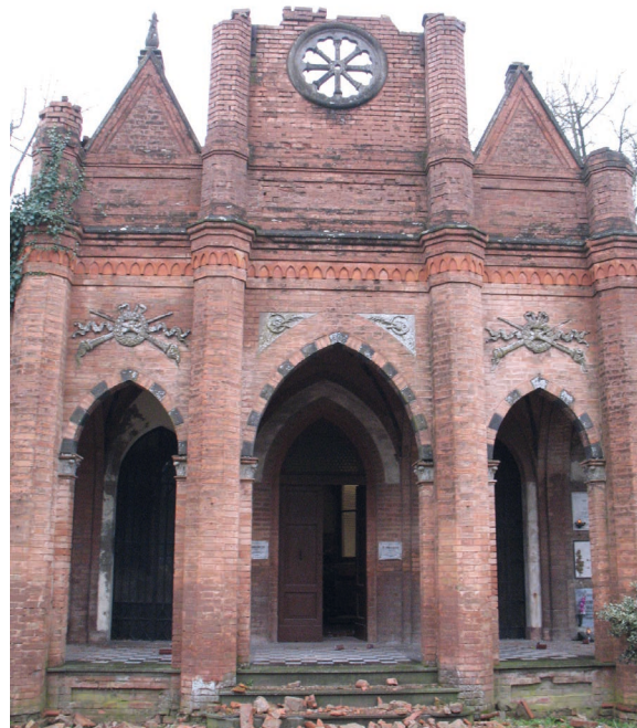
Fig.37. San Felice sul Panaro Cemetery. Collapse or damage of projecting elements of funeral chapels facades.
