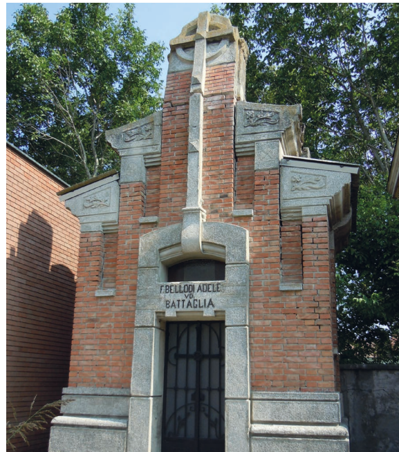
Fig.39. Cemetery of Vallalta (Modena crater area). Collapse of the projecting elements inside the family tombs.
