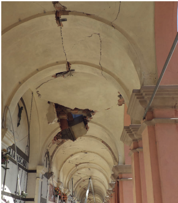
Fig.38. The Concordia sulla Secchia cemetery. Collapse of projecting elements inside the structures.
