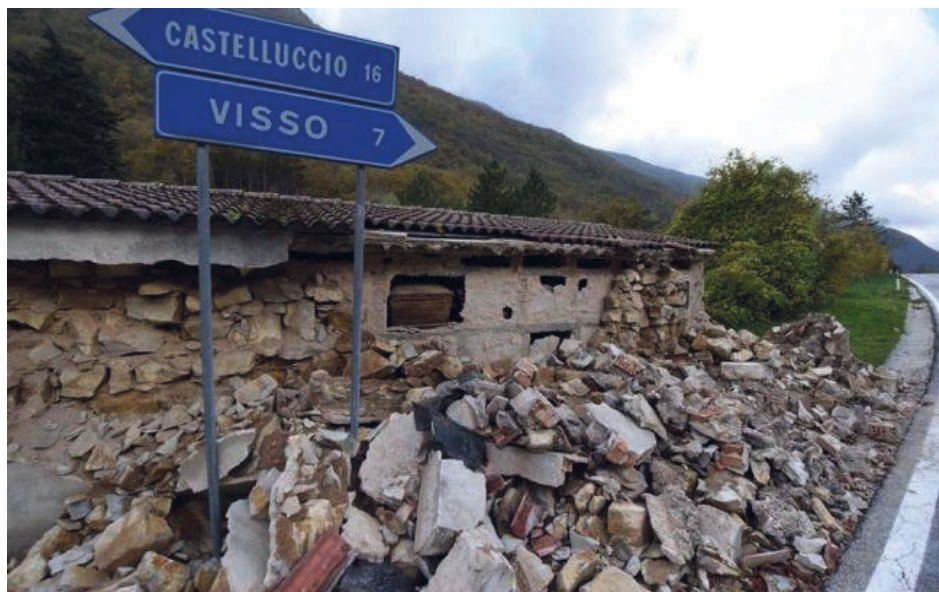
Fig.30. Image of the back wall collapse of the cemetery of Castelsantangelo sul Nera due to the absence of cross walls and poor construction quality. Source available at: https://www.cronachemaceratesi.it/2016/11/04/castelsantangelo-nelle-frazioni-annientate-il-terreno-piu-basso-di-20-centimetri/882095/
