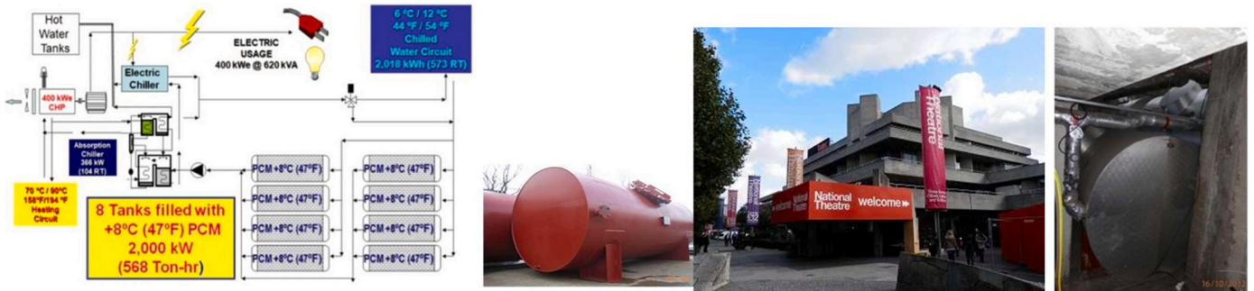
Fig. 10. Installed TES capacity, 8 storage tanks each with 8 \text{ m}^3 + 8 \text{ }^\circ\text{C} PCM solution providing total 2000 kWh [38].
