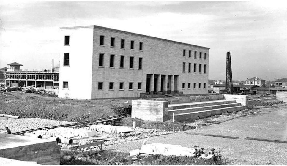
Figure 158. Photo taken during the construction of the campus of the University of Arts (source: AQTN)
