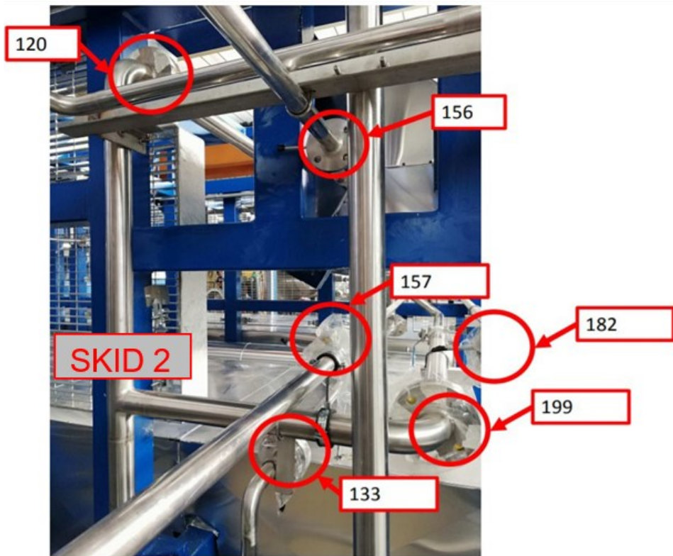
Figure 18: Blind flanges of skid 2 to be removed before the installation of skid 2 on skid 1. Interconnection lines between skid 2 and skid 3. Lines close to E-105
