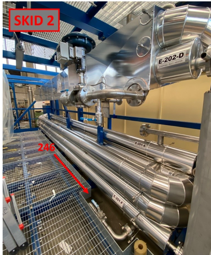
Figure 62: Blind flanges to be removed before the installation of skid 2 on skid 1
