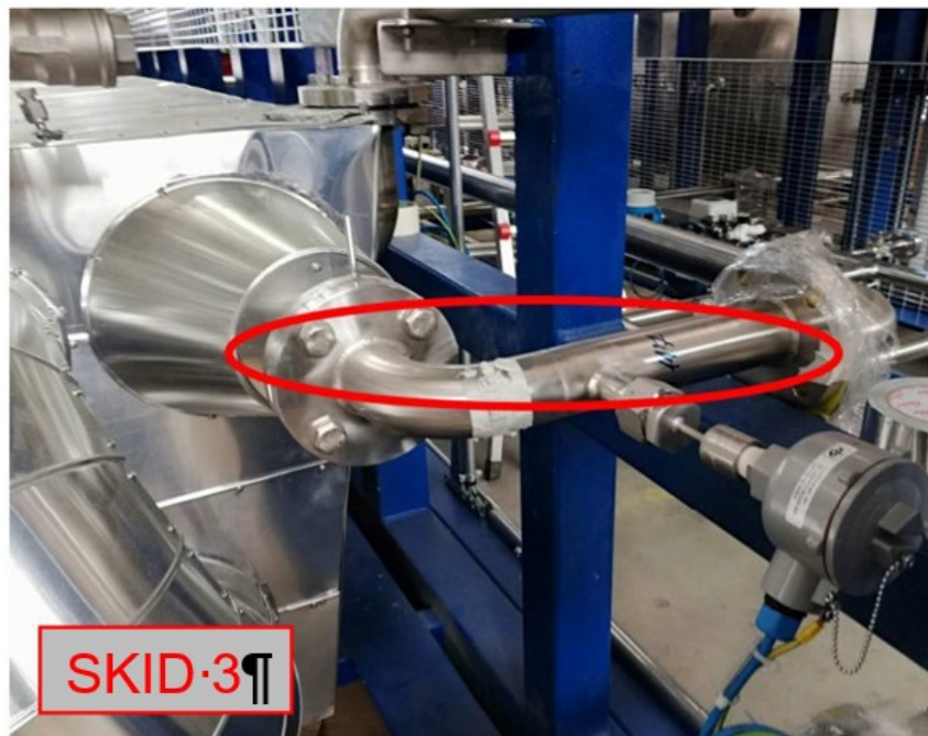
Figure 20: Blind flanges of skid 3. Line 169 connecting skid 2 and skid 3. It is composed by a removable pipe stub with a temperature transmitter mounted on (Pay attention to the temperature transmitter while removing the pipe stub).
