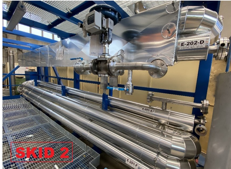
Figure 51: Location of E-201 and E-202 heat exchangers inside the Skid 2
