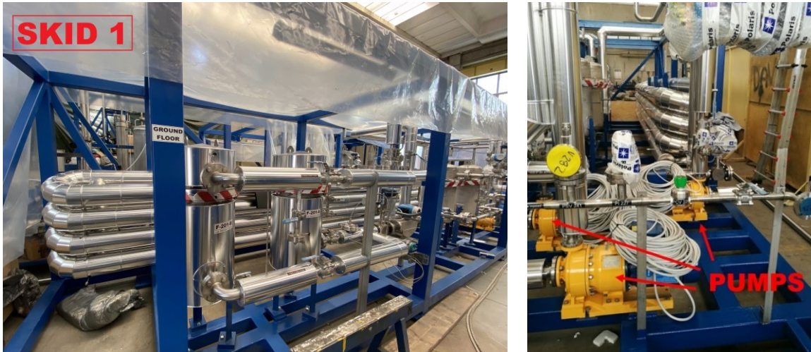
Figure 48: Skid 1 (left) and location of P-201, P-202, P-203 pumps (right) on skid 1
