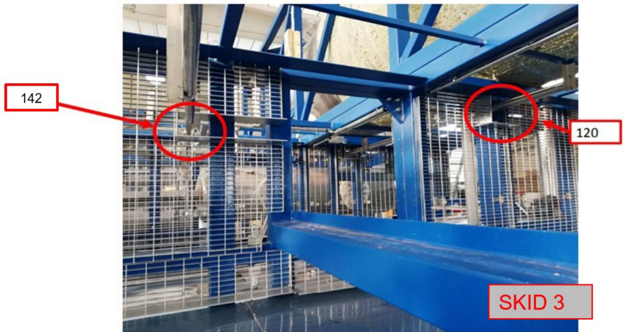
Figure 24: Blind flanges of skid 3 to be removed before the installation of skid 3 on skid 2. Interconnection lines between skid 4 and skid 3.
