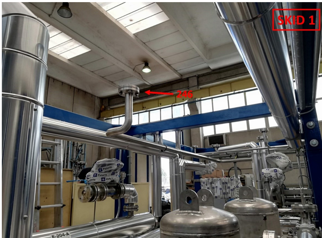
Figure 61: Blind flanges to be removed before the installation of skid 2 on skid 1
