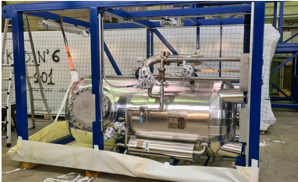
Figure 38: Blind flange on skid 5 for the connection with line 163
