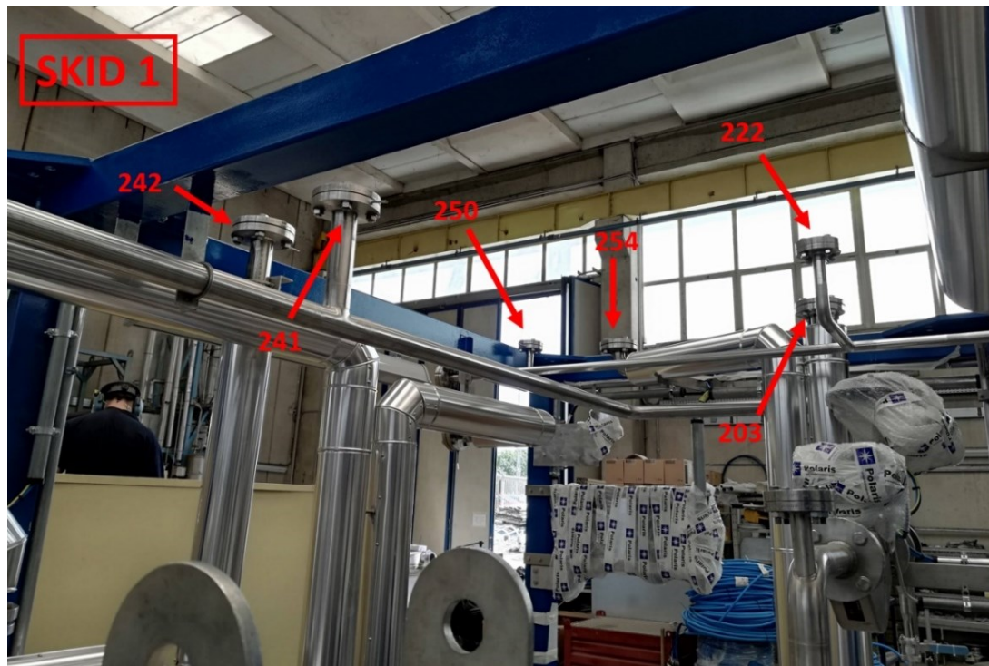
Figure 56: Blind flanges of skid 1 to be removed before the installation of skid 3 on skid 1. Leave the connection 241 and 242 with blind flanges on.
