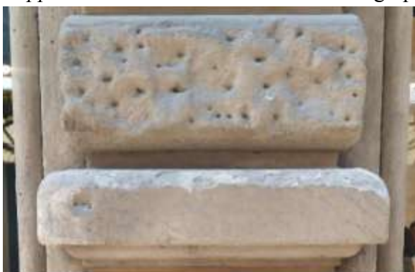
Fig. 1: The Bossage under study with evident damage due to flaking and exfoliation. Samples are taken from areas already decoached without further damage to the artwork
